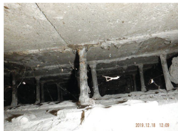
Figure 4: Exterior wall cavity with railroad track and ties.
