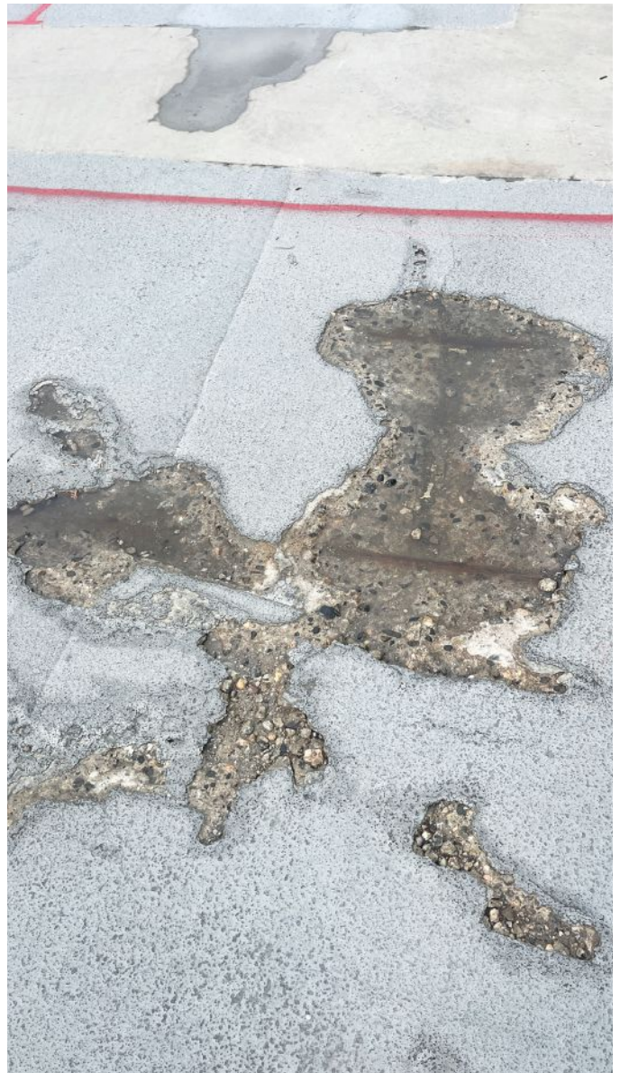
Figure 1: Suspected area of delamination.
