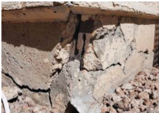
Figure 2: Typical rust jacked stem walls in the Southwest in corrosive conditions. Notice decorative landscape rock.
