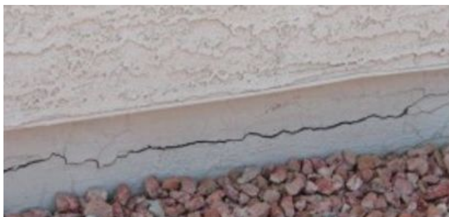
Figure 1: Typical rust jacked stem walls in the Southwest in corrosive conditions. Notice decorative landscape rock.
