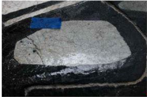
2 CRACK ID - C5
