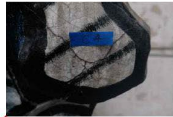
5 CRACK ID - C4
