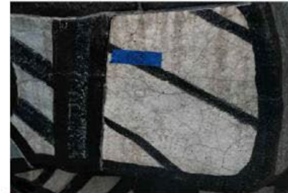
6 CRACK ID - C3 (2 of 2)
