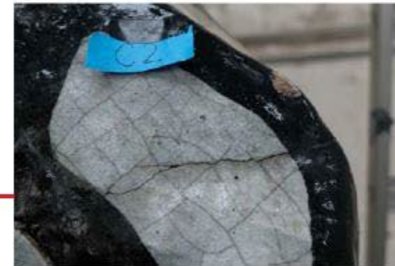
7 CRACK ID - C2
