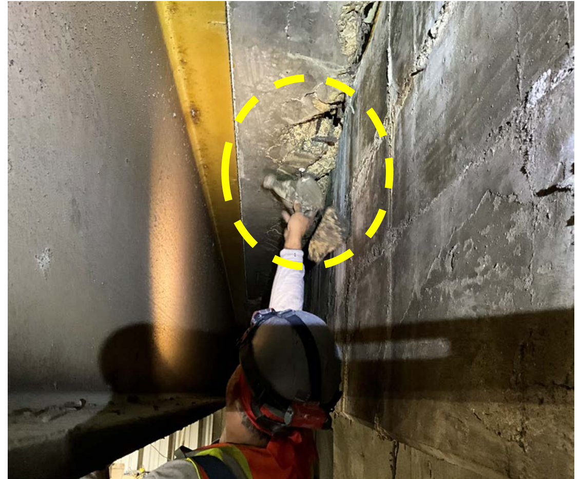
Loose overhead concrete
