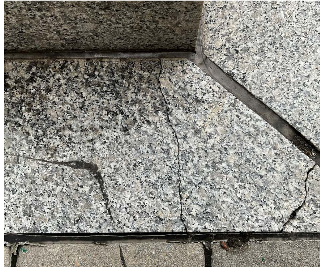
Cracked granite paver
