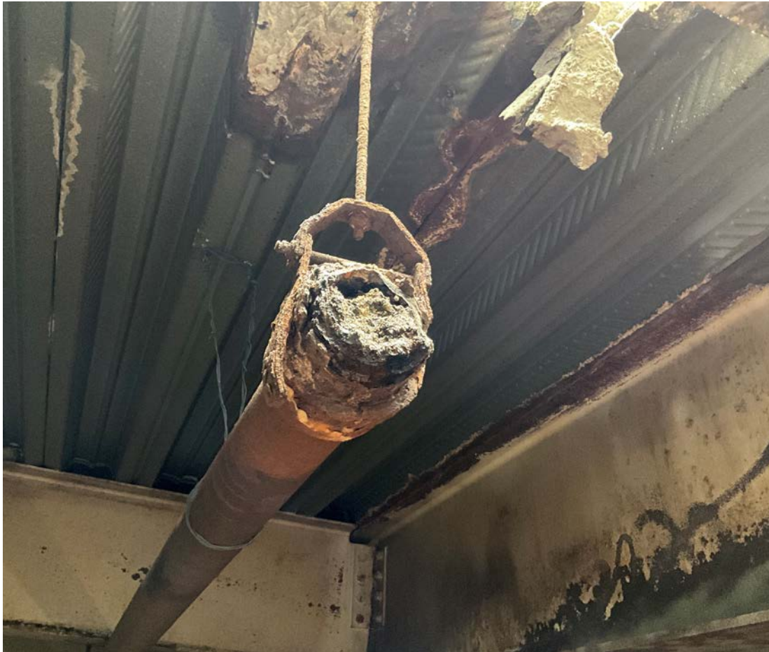
Drain pipe filled with sediment
