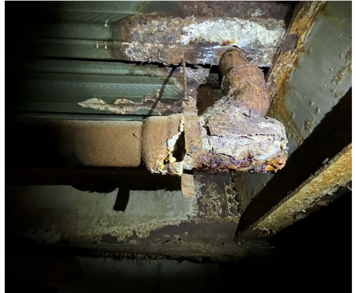
Corroded drain pipe
