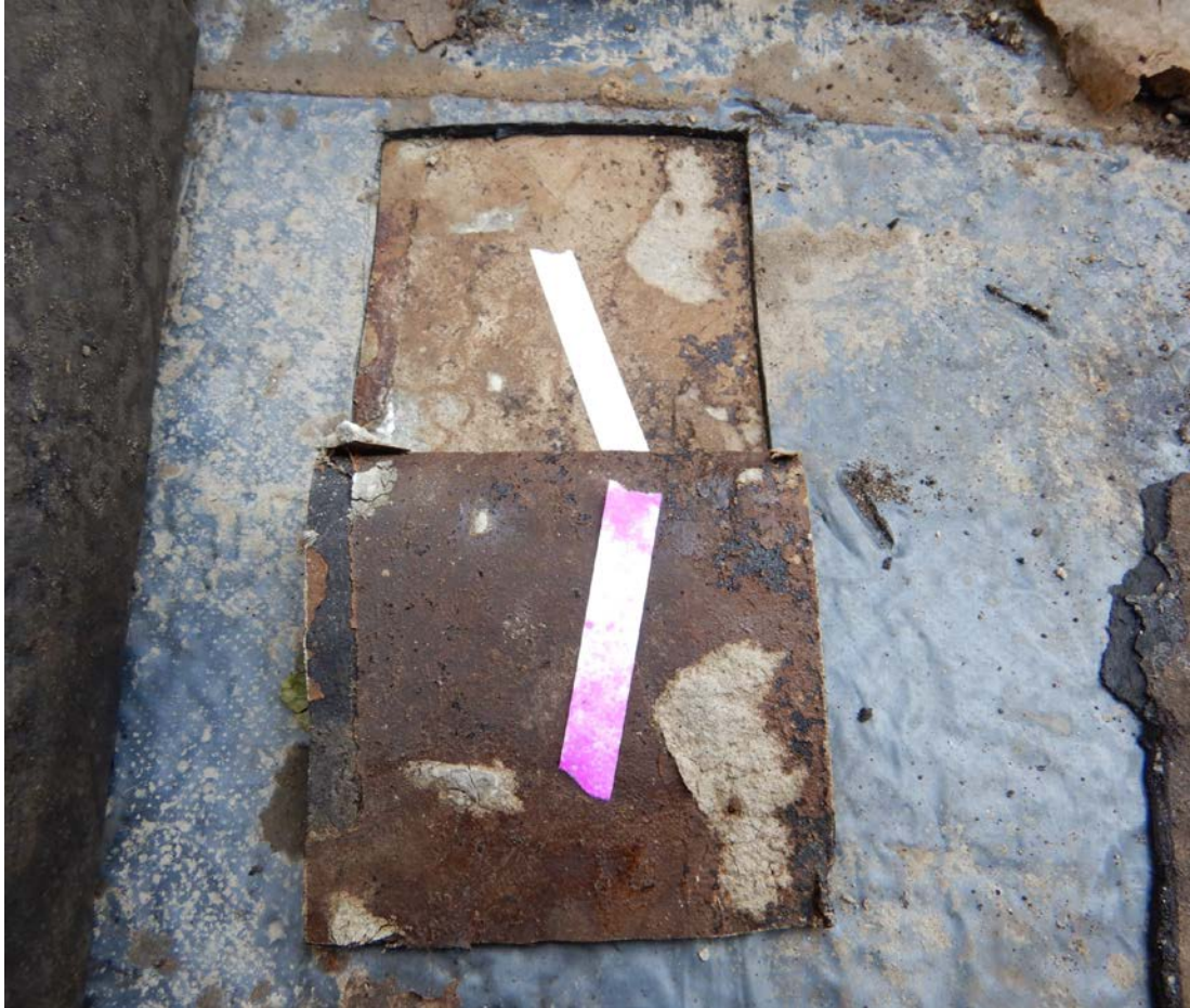
Water test paper, indicating moisture
