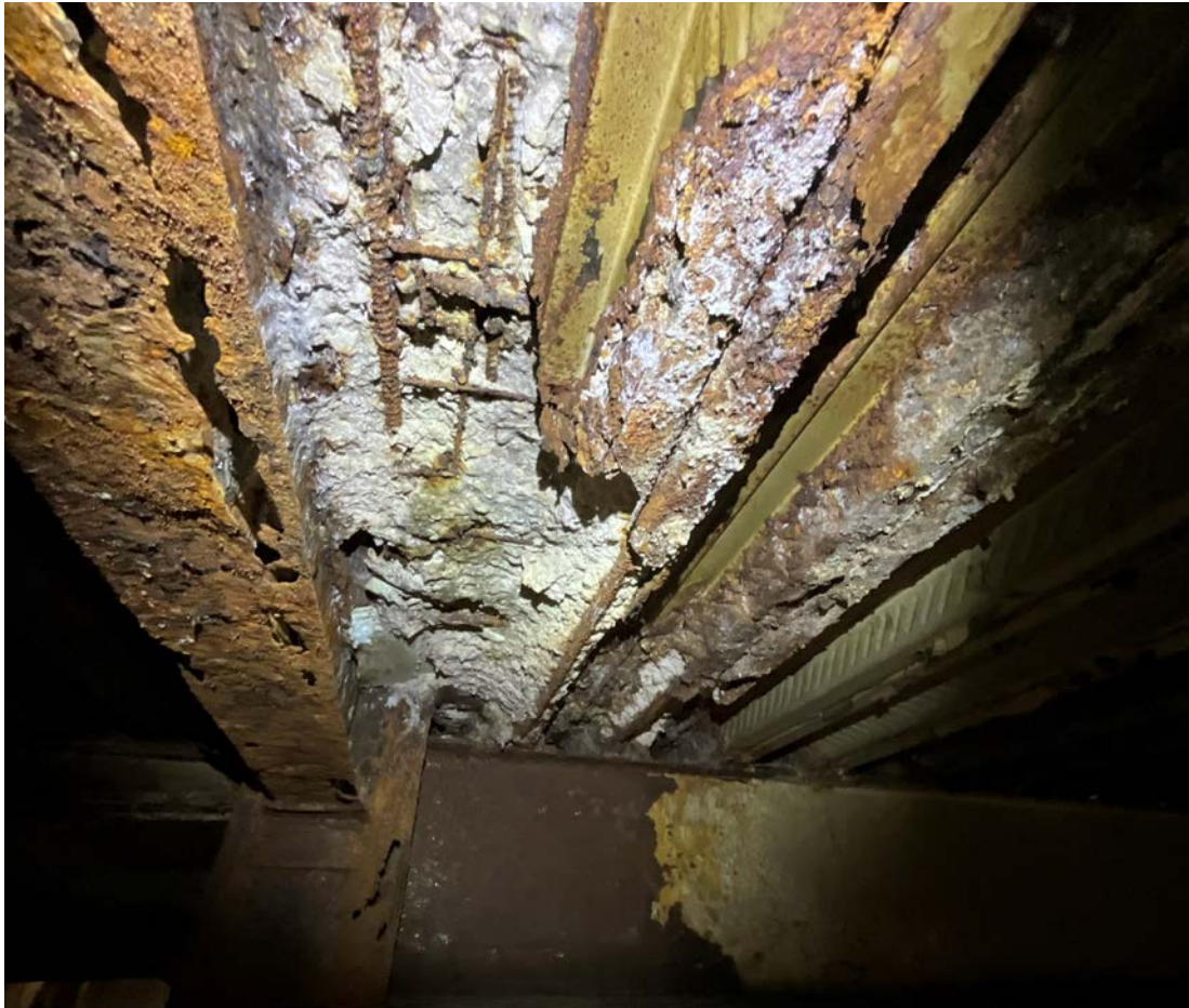
Corroded metal deck and deteriorated concrete
