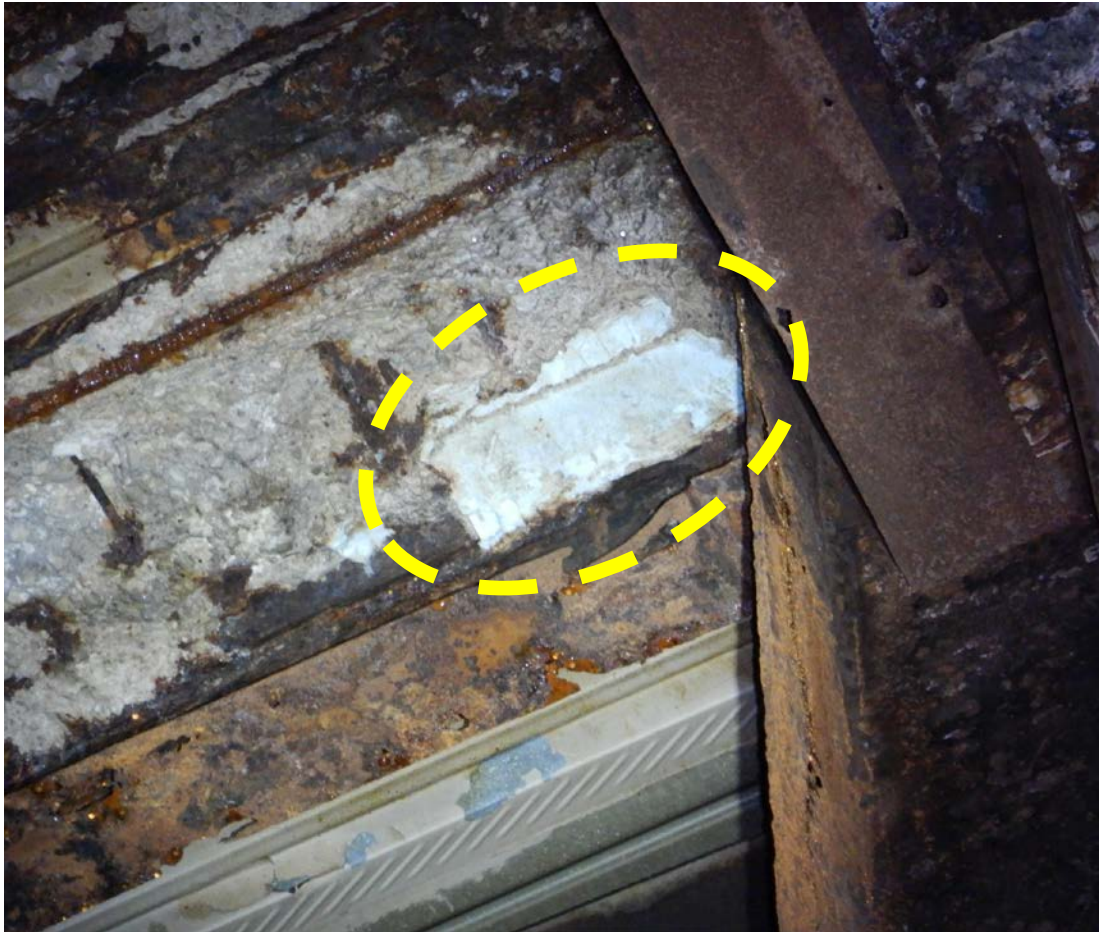
Hole through structural slab, rigid insulation at bottom of planter visible
