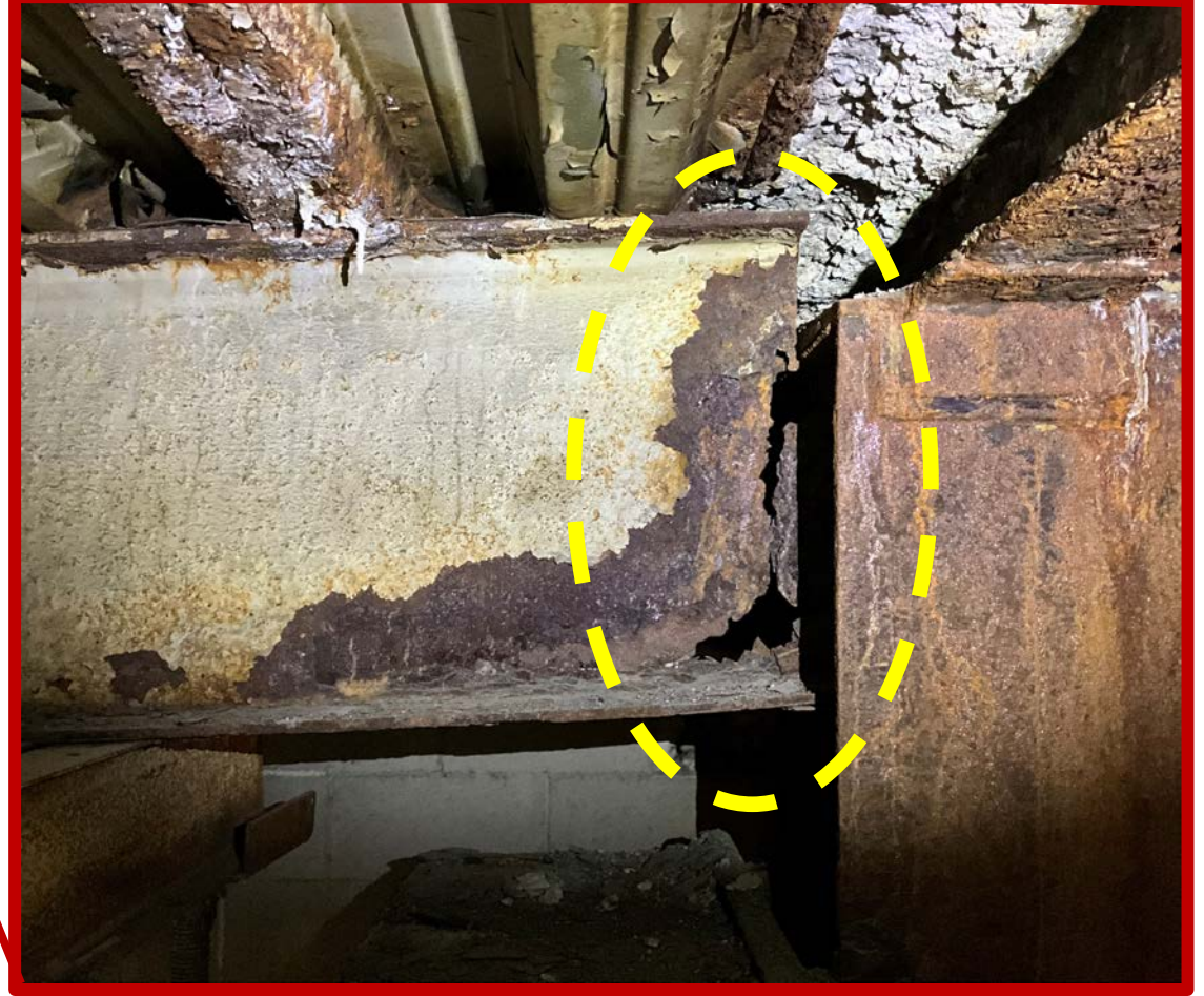
Completely corroded steel web and sheared-off beam-to-column connection
