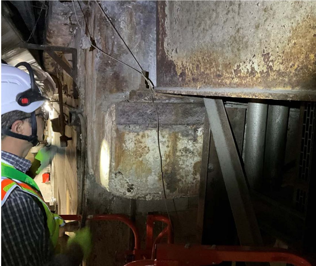
Deteriorated corbel and corroded baseplate
