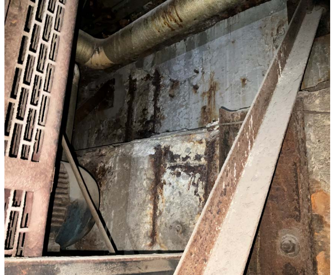
Exposed reinforcing behind generator
