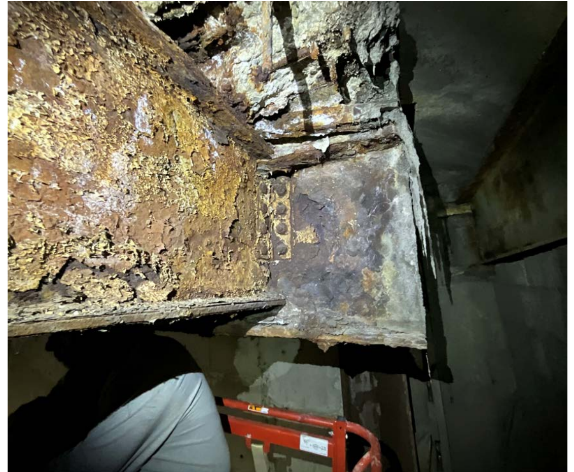
Corroded steel beam
