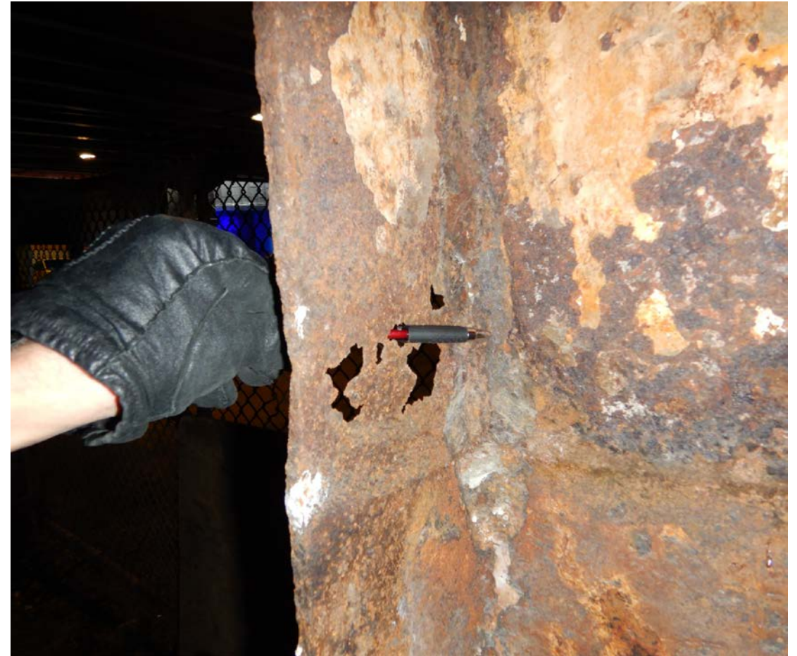
Hole through a column flange
