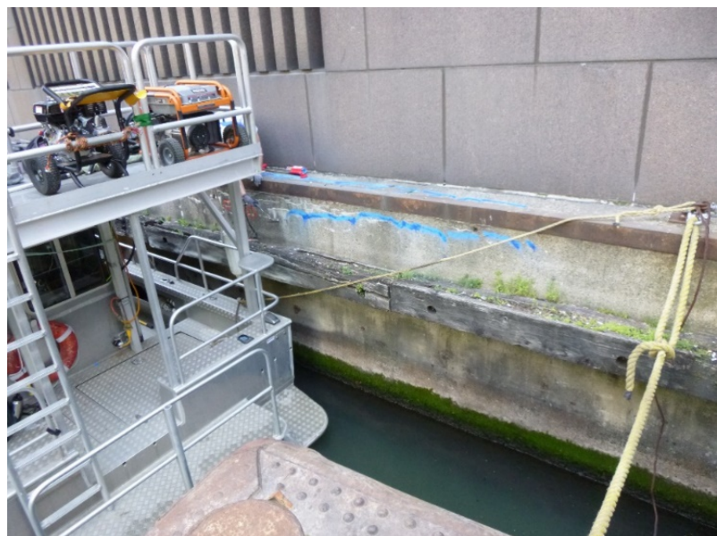
Overall view of sheet pile retaining wall structure above the water level
