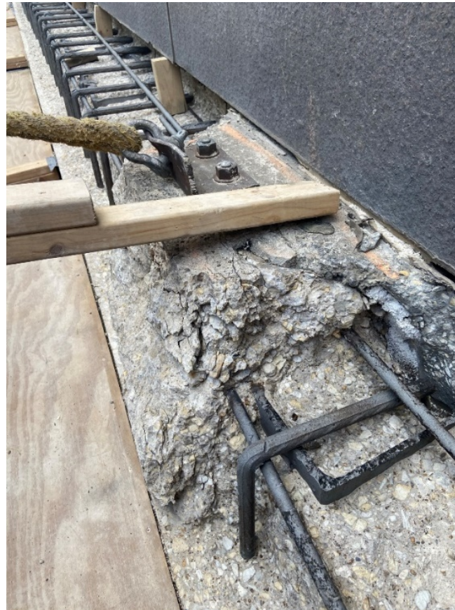
Section of delaminated concrete at the wall cap where boat tie-off is used for the barge
