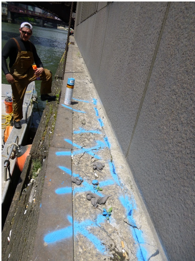
Concrete distress across the full width of the top surface of the cap
