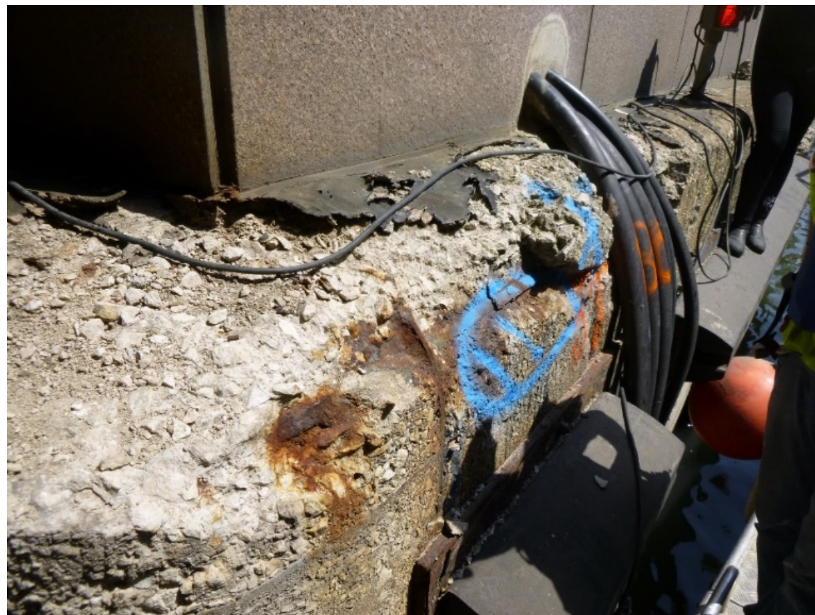
Spalling on top of timber pile river wall (City's property)
