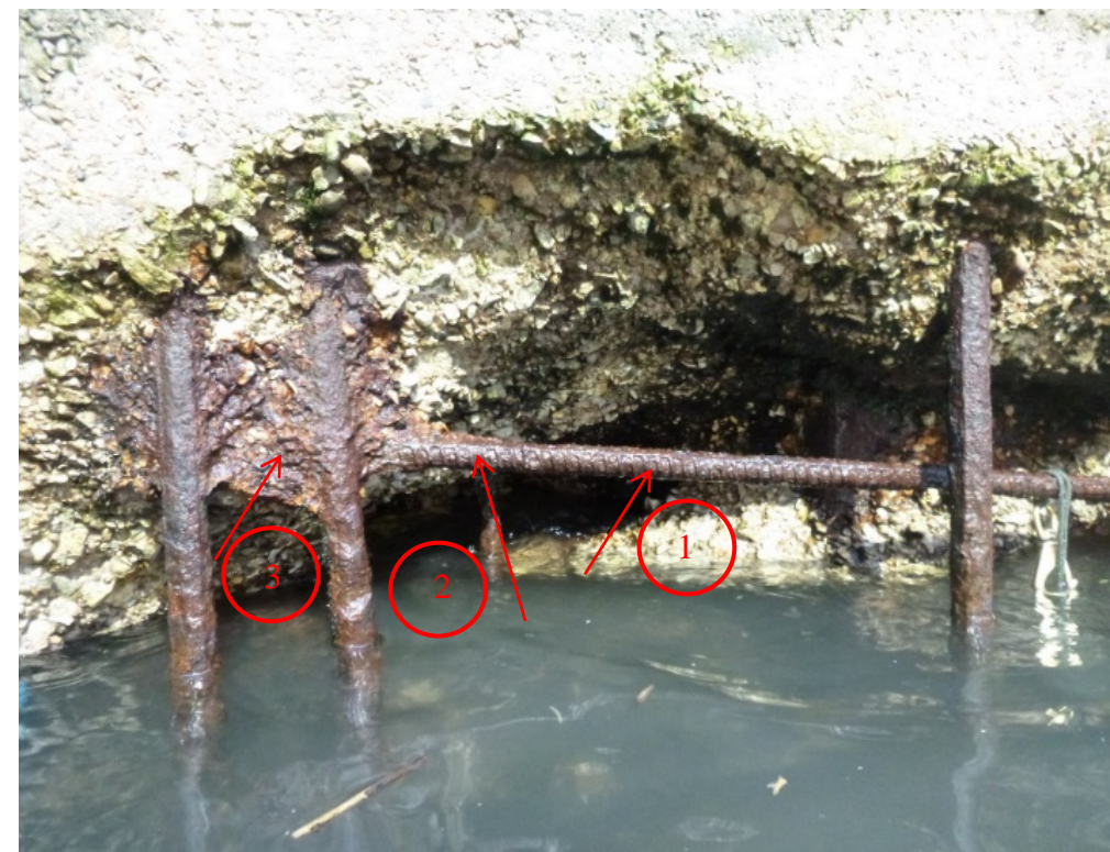
Spall at waterline exposing inside face of sheet piling
