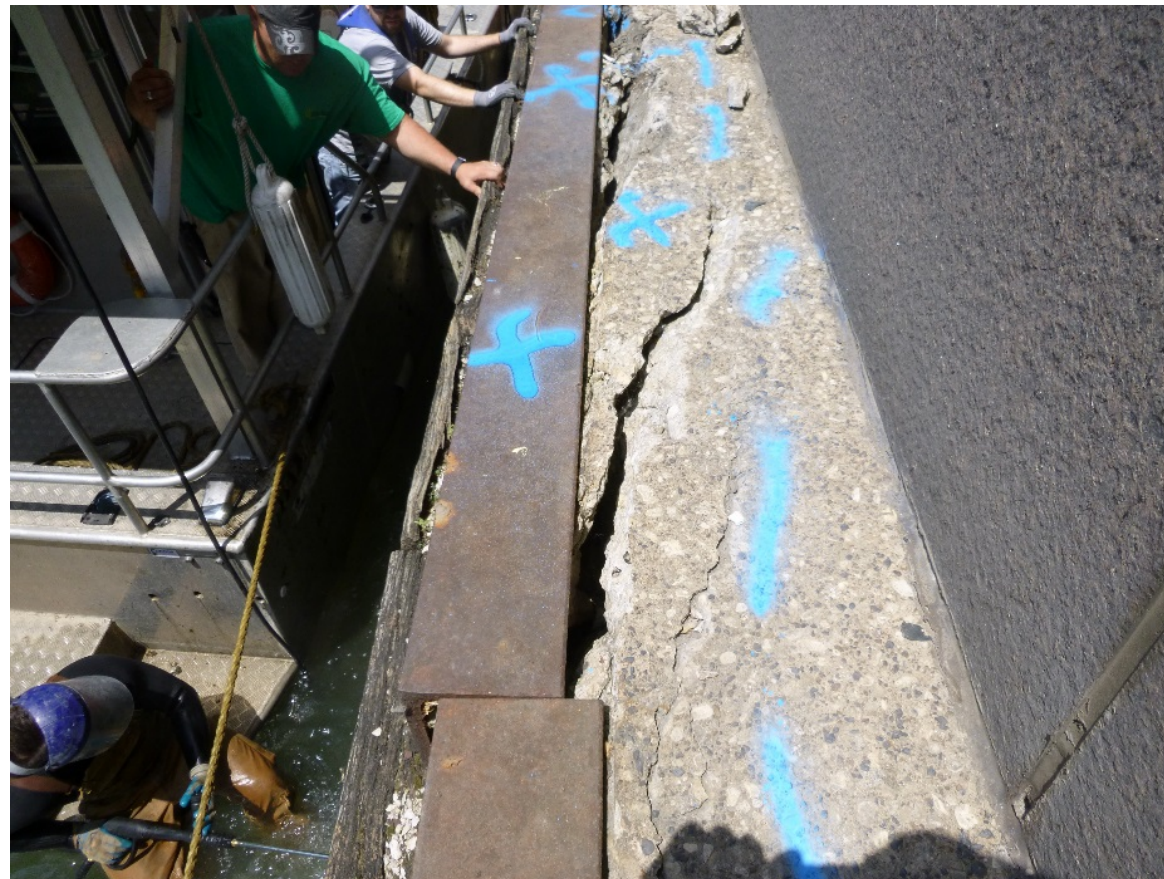
Spall behind angle at Station 2+30
