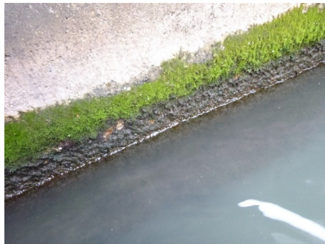
Surface erosion and marine growth at bottom of concrete cap
