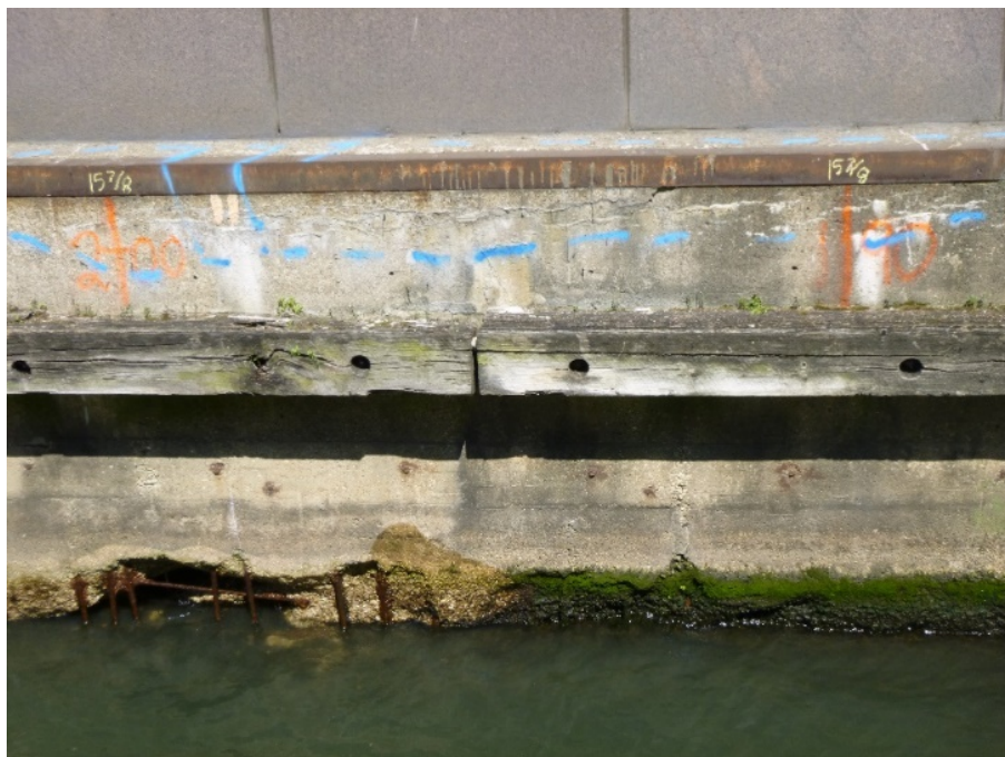
Typical concrete distress (outlined in blue paint) at top of concrete cap
