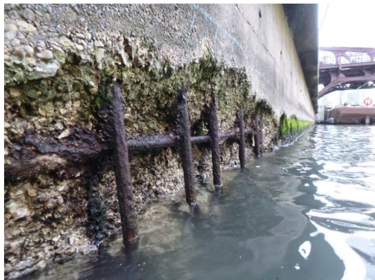
Severely eroded concrete at waterline
