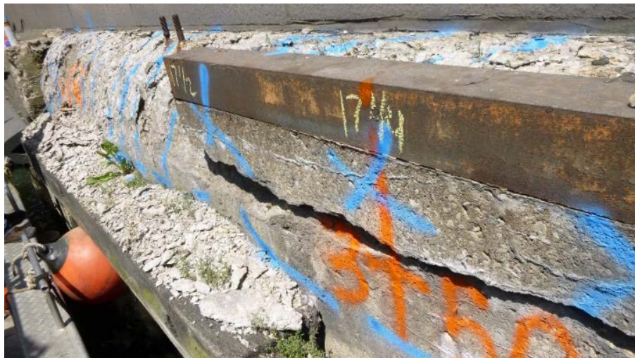
Concrete spall between Station 3+50 and Station 3+60
