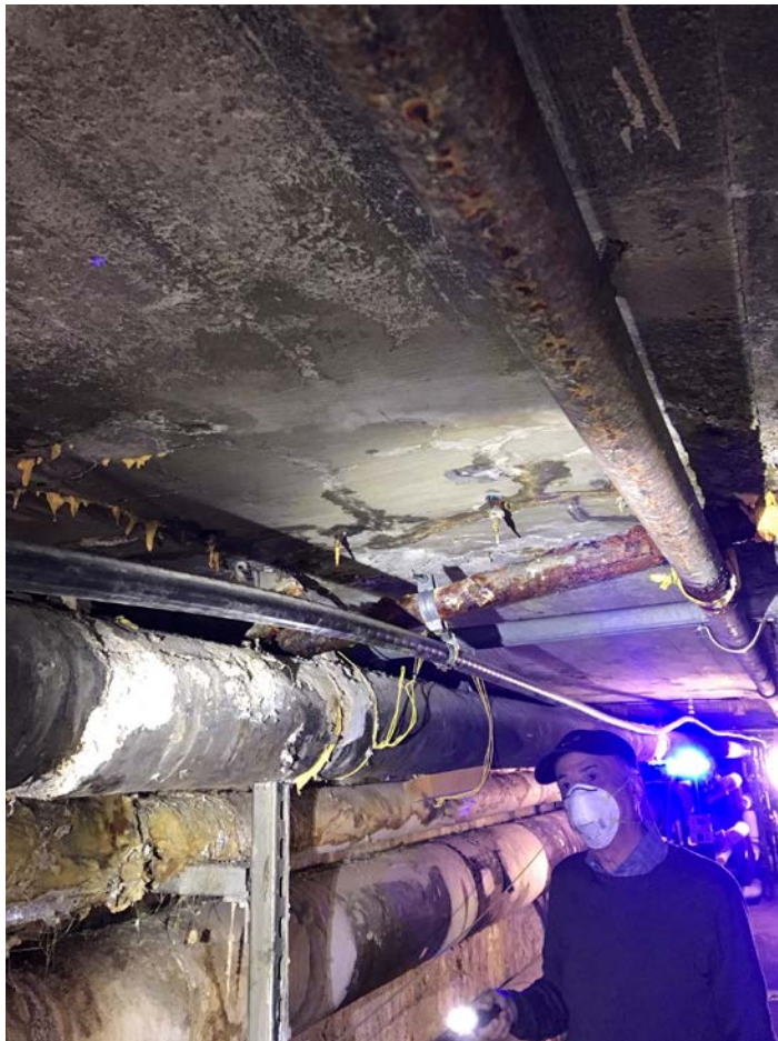
Injected cracks in good condition, new ones have formed
