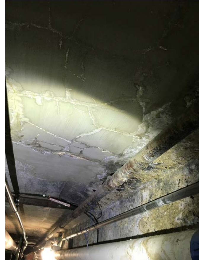
Larger overhead repaired areas with leaking cracks but sound
