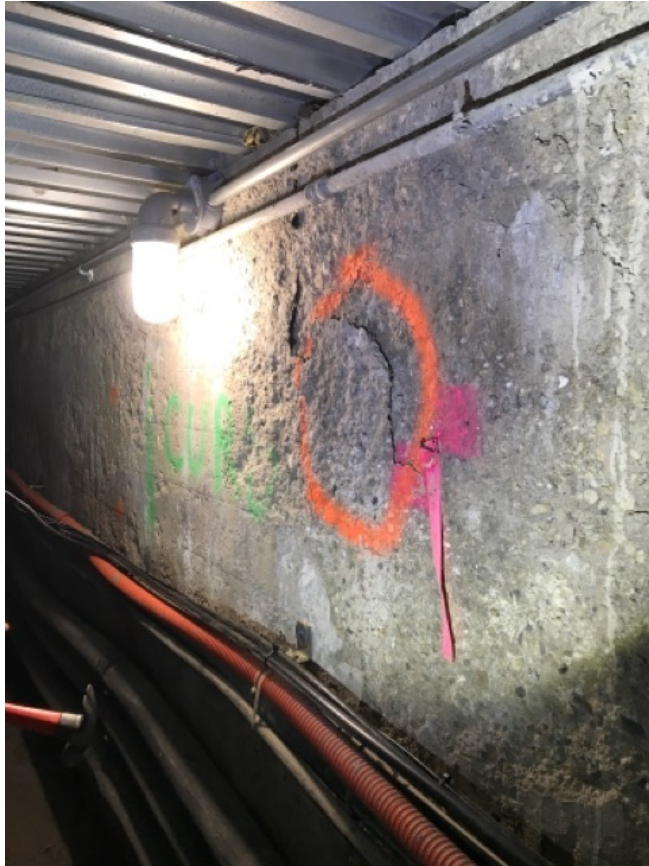
New spalls observed at small number of locations
