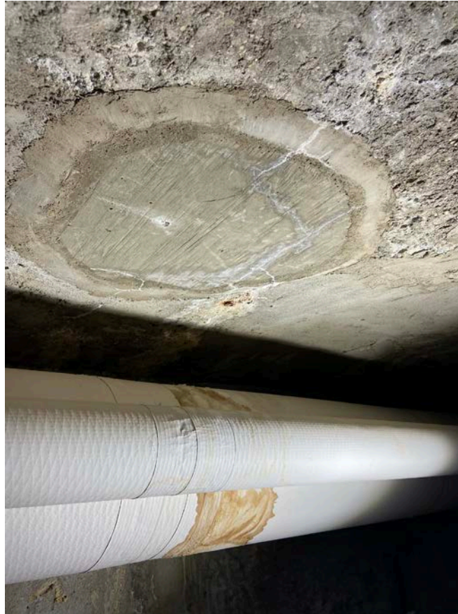
Small overhead repaired areas with leaking cracks but sound
