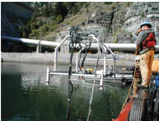
Fig. 9: Hydrodemolition cutting frame being lowered to basin floor at 50 ft (15 m) below the surface
