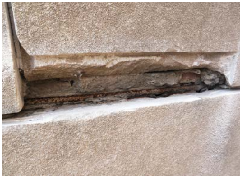
Fig. 3: Corroded steel relief angle
