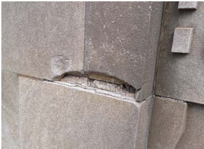
Fig. 2: Spalled stone observed during condition survey of façade
