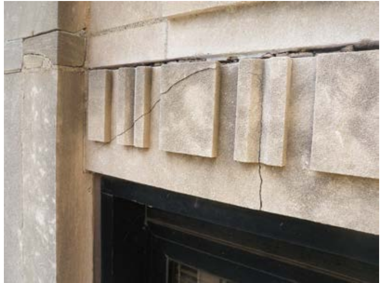
Fig. 7: Cracking in stone panel above window head
