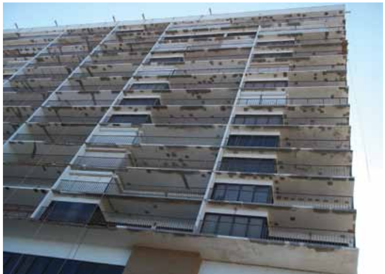
An extensive amount of concrete repairs were required for the balcony edges and soffits
