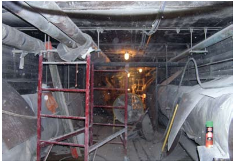
Example of the conditions in the tunnel at the beginning of the project
