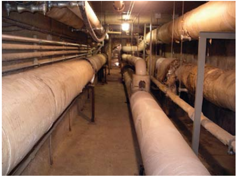
View of a completed segment in the tunnel showing new steel pipe supports and hangers, repaired concrete surfaces, repaired steam pipe insulation, and new lighting
