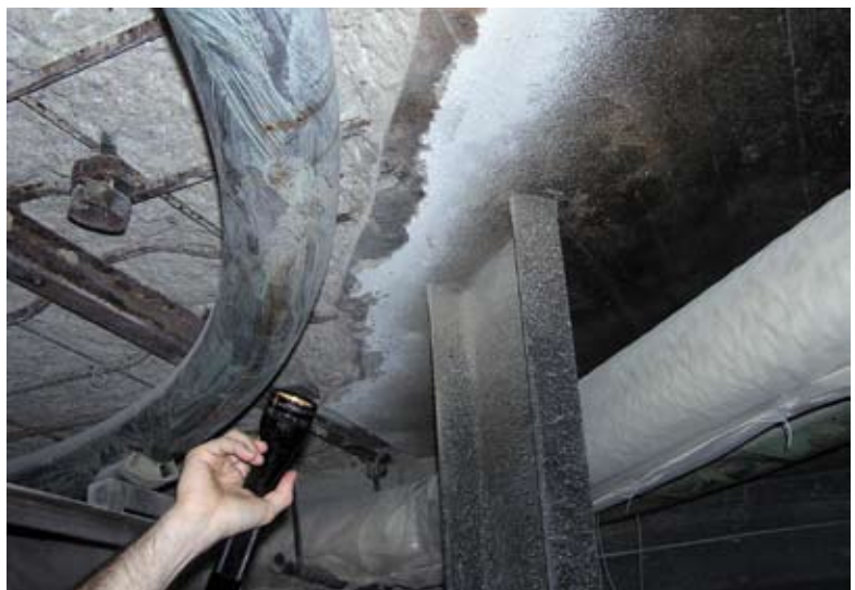
Another example of the existing conditions that restricted access to the concrete restoration areas
