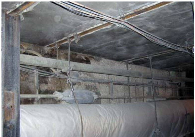
Difficult-to-access deteriorated concrete behind steam lines and above exposed loose communications wiring
