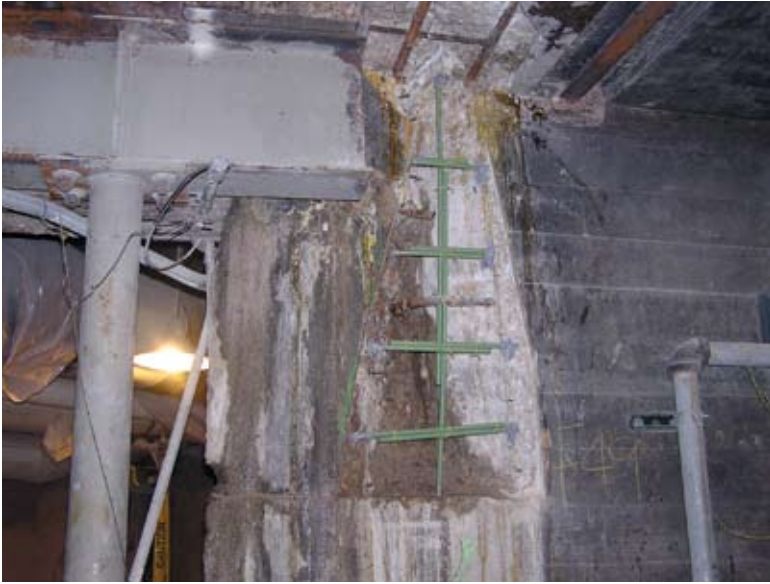
Damaged concrete wall during preparation and a new supplemental steel beam with columns
