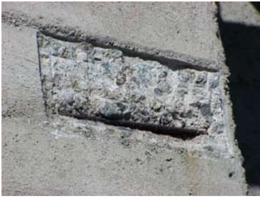
Close-up of spall prior to repair
