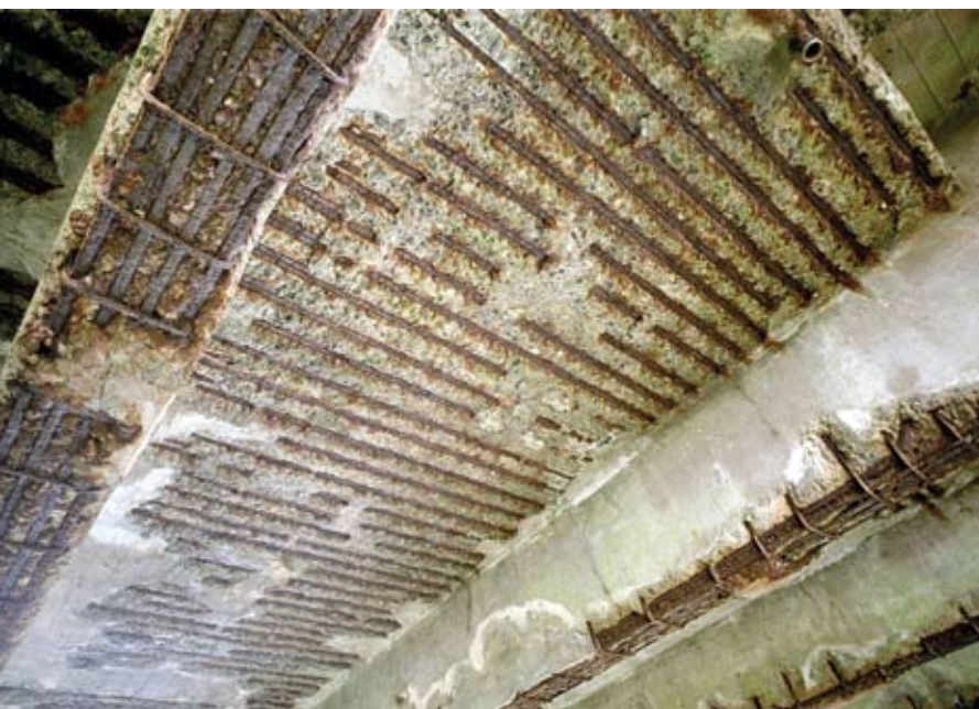
Corroded reinforcing steel in concrete deck
