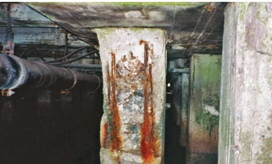
Corroded reinforcing steel in concrete pile
