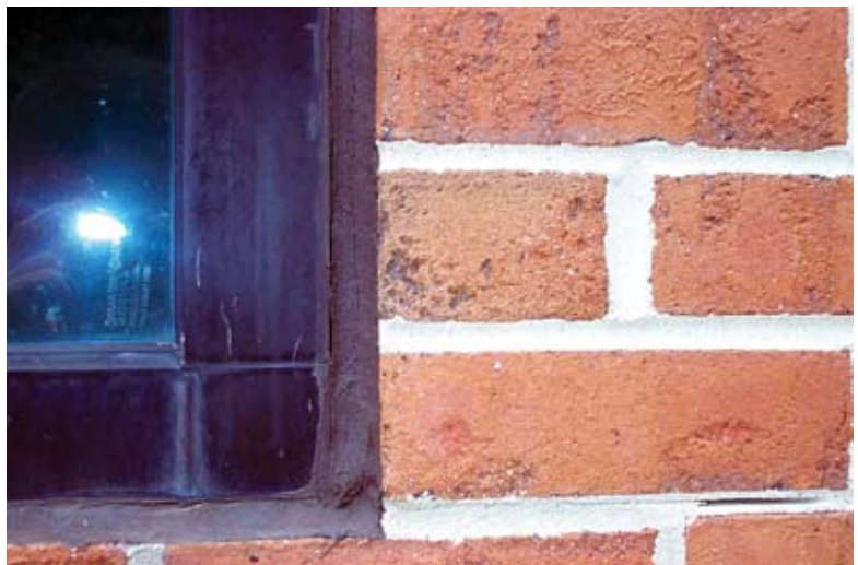
Improper adhesion of sealant on window due to poorly formed joint. Bonding area on metal is insufficient to provide adequate sealant bond
