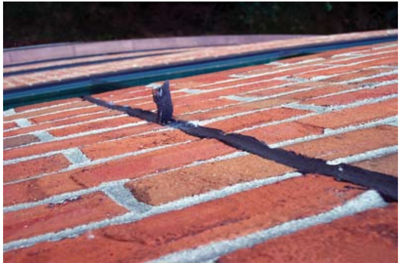
Control joint improperly installed with new sealant applied over old sealant. Note how new sealant can be pulled off old sealant
