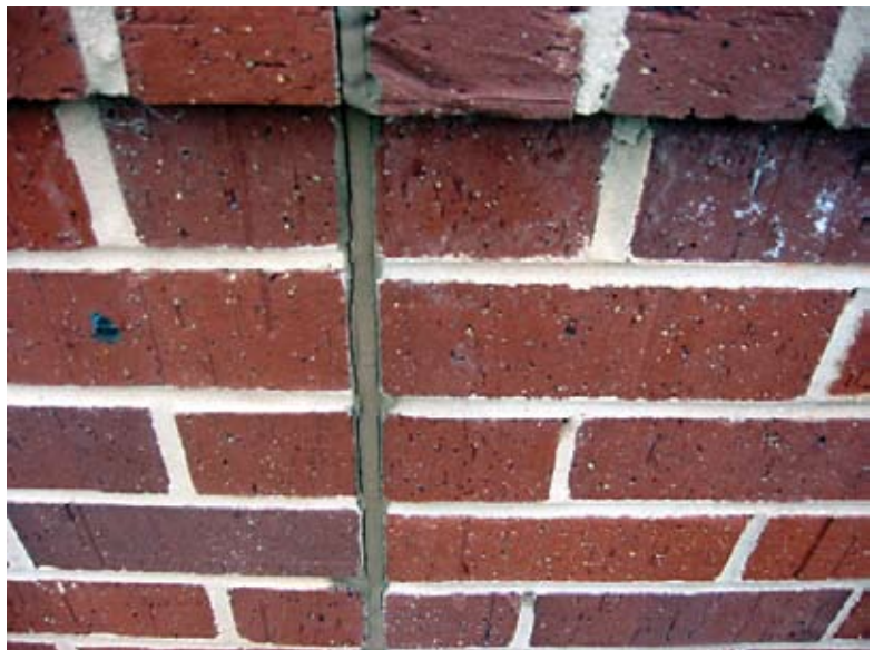
Adhesion failure of sealant on masonry joint. Improper preparation and lack of primer can cause debonding
