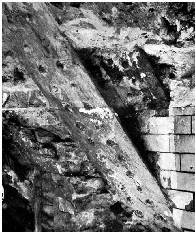
Fig. 1: Early 20th century steel frame showing corrosion, as reported in 1947
