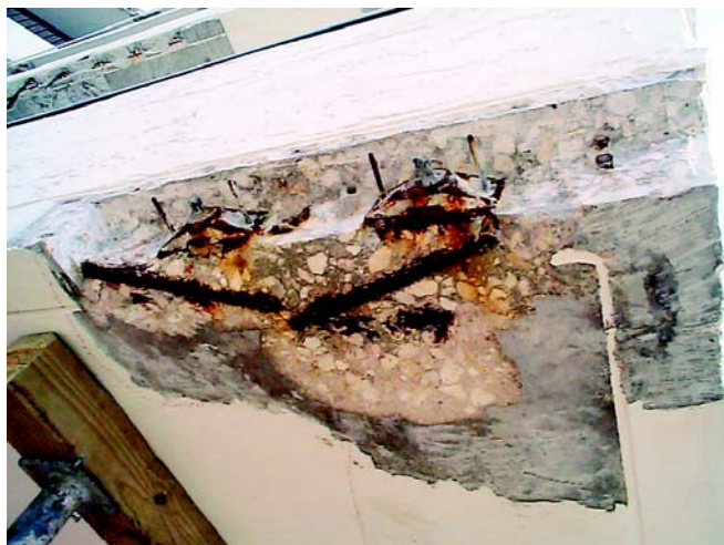
Anchors with spalled concrete exposing corroded bursting bars
