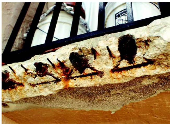
Close-up of balcony slab edge with spalled concrete exposing corroded bursting bars
