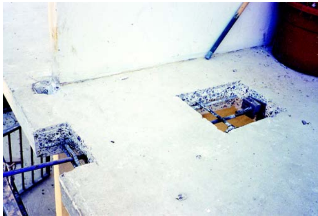
“Text book” repair of slab edge (Note the temporary lock off and slab edge with excavation per ICRI guidelines)
