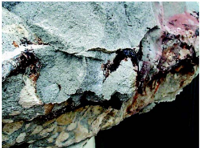
Improper slab edge repair that has failed (Note new mortar on top, old substrate below, and bursting bars sandwiched between)
