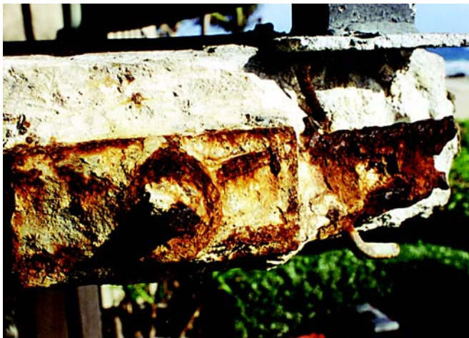
Anchor with spalled concrete exposing corroded bursting bars
