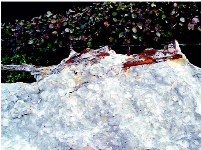
Anchor that is still under tension and has burst out of concrete during repair demolition
