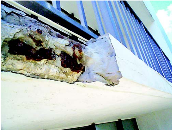
Improper slab edge repair that has failed (Note bursting bars and anchor are sandwiched between new mortar and old concrete)
