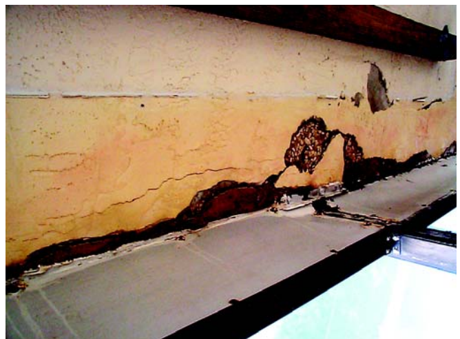
Balcony slab edge showing previous repairs that have failed and are spalling
