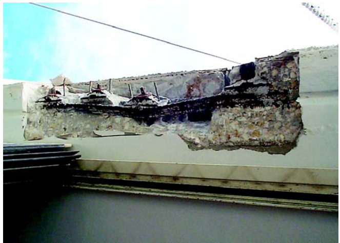
Top edge of slab showing improper repair demolition (Note corroded reinforcing steel and cracks in concrete behind anchor)
