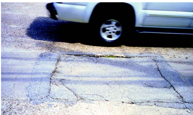
Failure of pavement patch
