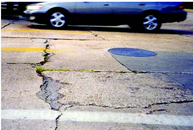
Severe cracking of pavement and patch
