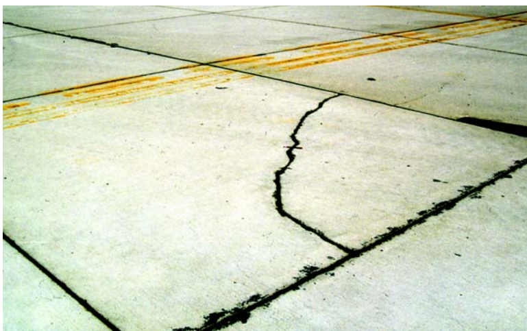
Common pavement crack pattern
