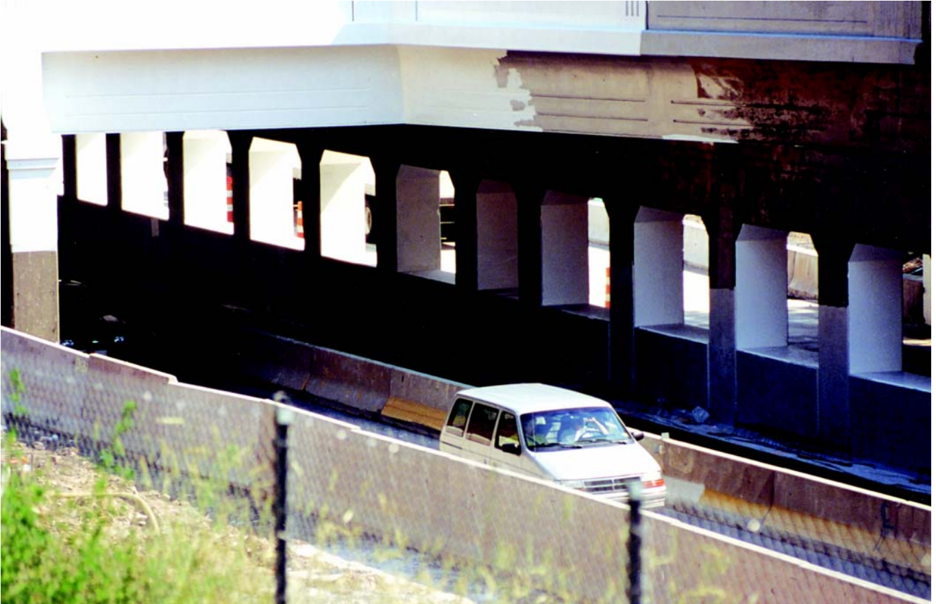
The façade of this bridge along Pennsylvania State Route 322 was coated with a high-performance urethane primer/coating system to protect it from graffiti and unify its appearance
