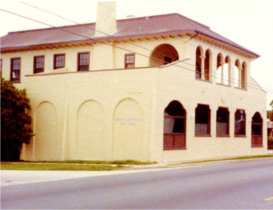
Following repair and restoration of the concrete façade, the South Daytona City Hall in Florida was coated with a urethane primer/coating system to upgrade the aesthetics and protect it from the effects of ultraviolet rays
