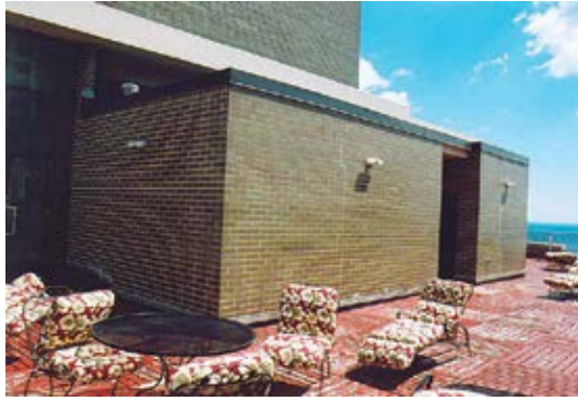
View of south sundeck prior to repair project; north sundeck is identical
