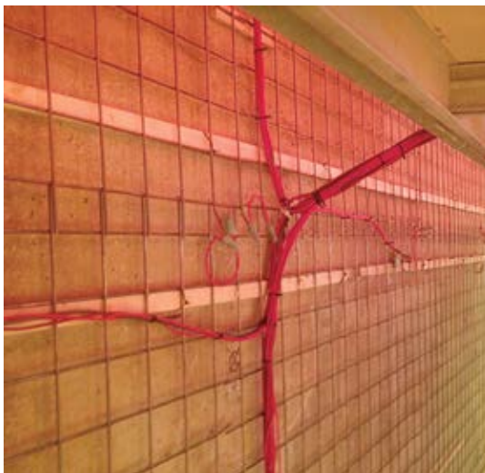
Temporary anode mesh and wiring in place for electrochemical chloride extraction treatment for the two land-based piers
