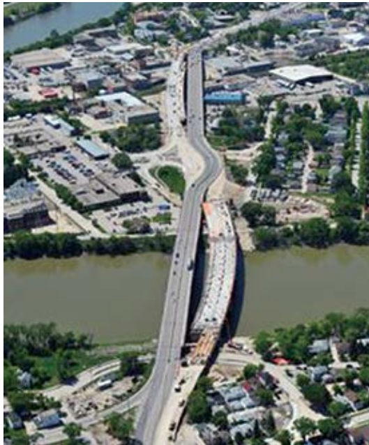
Aerial view of the Disraeli Bridges project over the Red River with traffic diverted onto the new bridge
