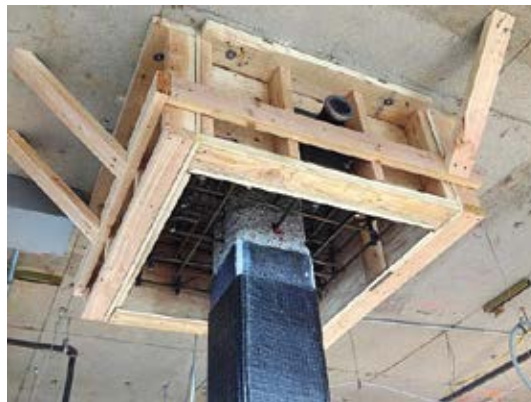
Column capital enhancement and full column wrap with a composite strengthening system for axial strength
