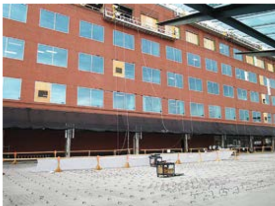
Prior to placement of concrete, reinforcement of the bonded overlay was performed on the transportation area deck
