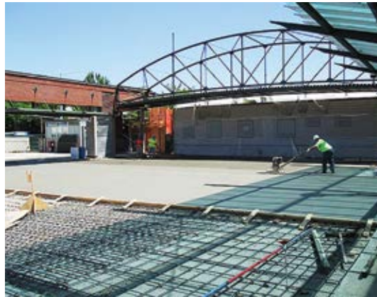
Placement of bonded overlay over the parking structure created a strengthened deck for the public transportation area
