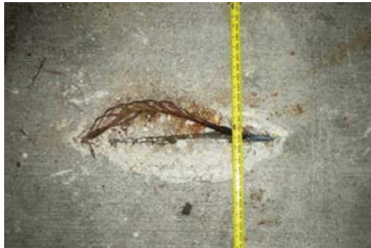
Fig. 2: Post-tensioned tendon failure
