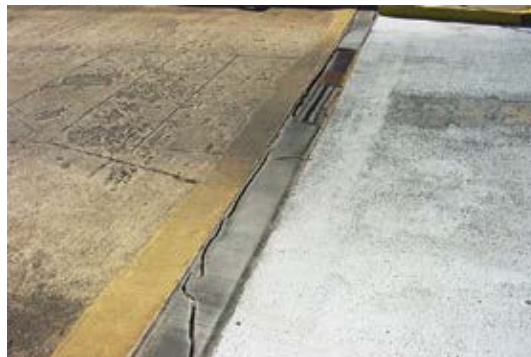
Fig. 1: Expansion joint failure
