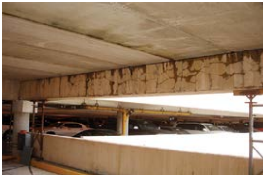
Fig. 3: Deteriorated bridge beam (inside face)
