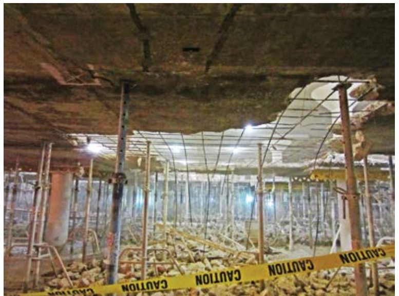
Lower-level shoring and reshoring due to unforeseen conditions
