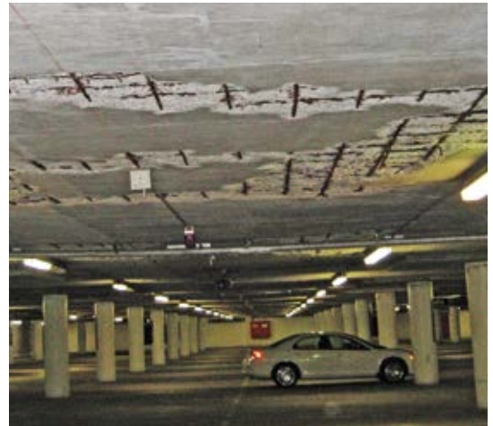
Existing ceiling of the lower level prior to repair
