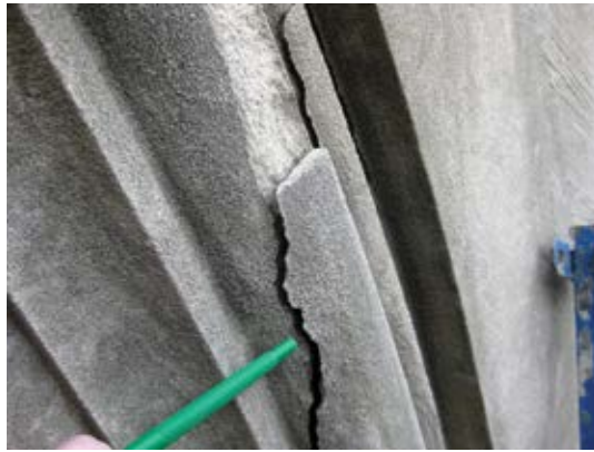
Damage to medallion
