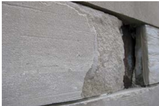
Damage to ashlar unit
