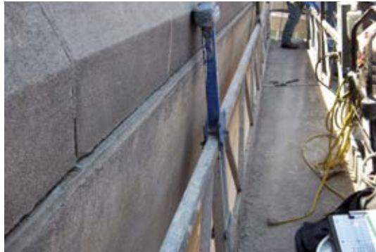
Displacement of large parapet and coping units
