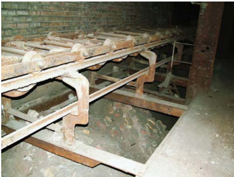
Existing coal conveyor boiler feed system
