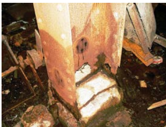
Deterioration of existing column section
