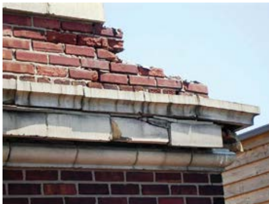
Typical deterioration of exterior brick and terra cotta cornices
