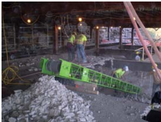
At the interior levels, debris was removed from the scaffold platform using conveyor belts and hauled to dumpsters using a small skid steer
