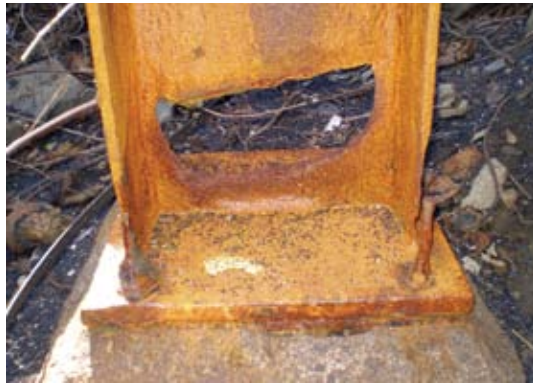
Erosion of the steep hillside on the west side of the structure had buried several column bases and beams, causing the soil to hold moisture and cause deterioration
