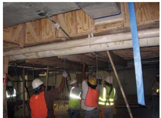
Workers installing the formwork suspended from the slab above that allowed existing utilities to remain in place during strengthening
