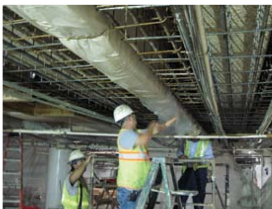
Workers installing reinforcing steel for section enlargement and distribution ribs with existing utilities still in place
