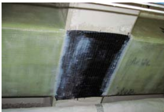
Installed CFRP on bottom of beam for flexural reinforcement and GFRP U-wrap for shear reinforcement
