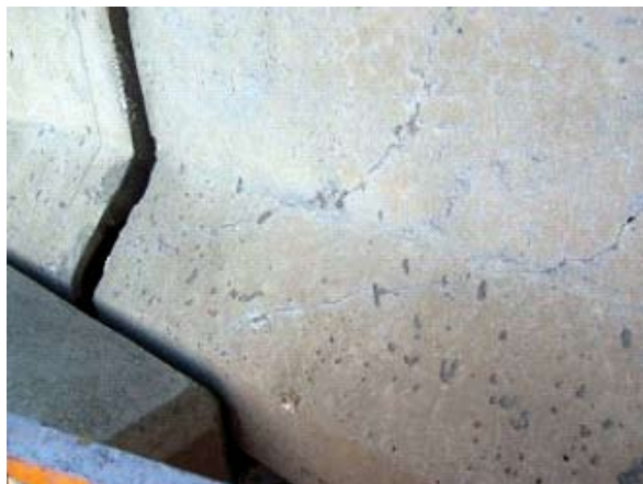
Typical shear cracks
