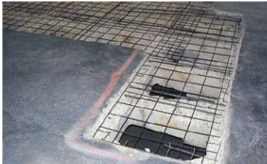
One of the parking garage full-depth slab repairs, prior to installation of zinc anodes for galvanized cathodic protection. At this phase in the repair, zinc anodes were attached to the reinforcing steel and wire mesh system along the perimeter of the repair area
