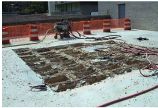
A large portion of the top level of the parking garage experienced deterioration due to poor drainage. This slab was repaired in one large deck repair and was finished with the proper slope to permanent drains, which allowed the contractor to eliminate several of the existing drains and improve the drainage of the top level parking deck
