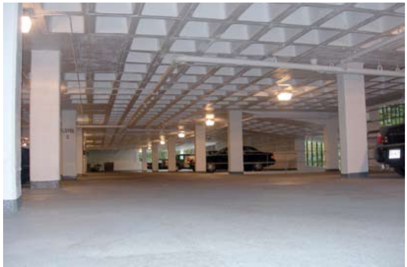
Concrete repairs using galvanized cathodic protection, protective traffic bearing coatings, and painting of columns, walls, and ceilings were performed in the five-level parking garage
