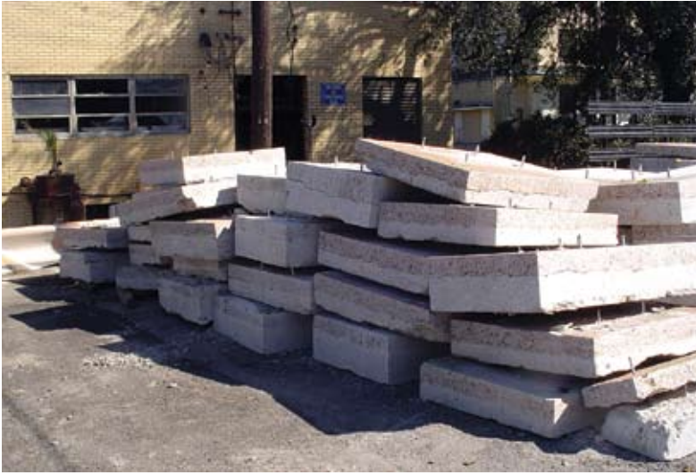
Concrete blocks stacked after being saw cut and removed from dock slab
