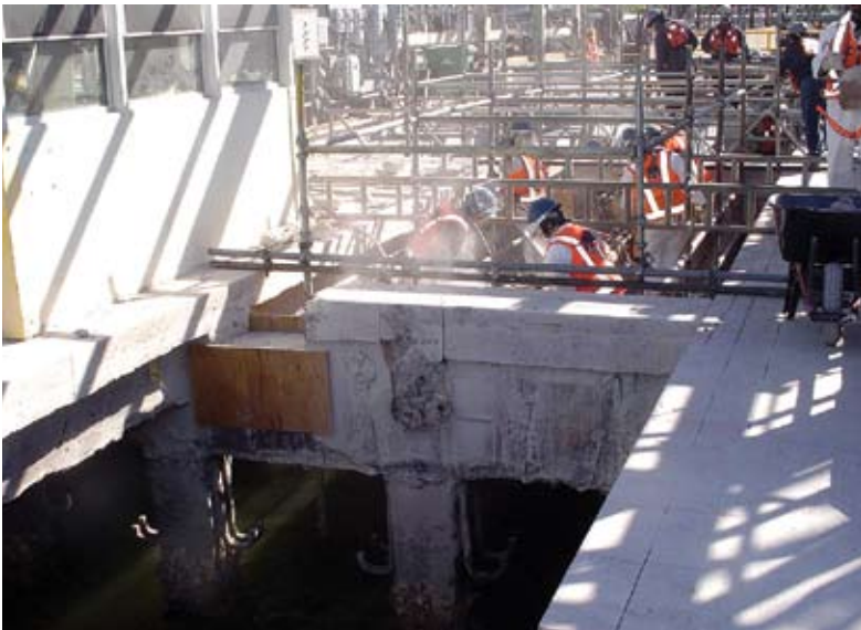
Crews removing intermediate beams using pneumatic chipping hammers; due to the thickness of the beams, they could not be safely removed by saw cutting
