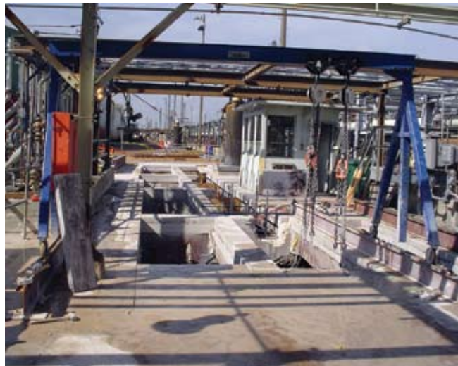
Concrete slab demolition; blue A-frame with chain hoist was used to lift out concrete blocks after they were saw cut
