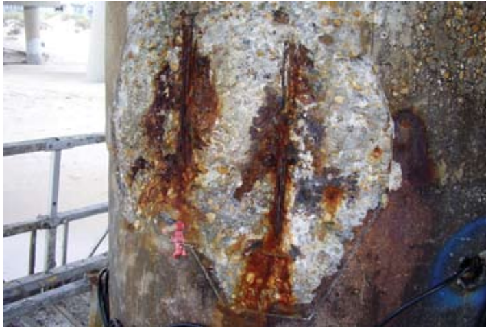
Corrosion of vertical pressed steel
