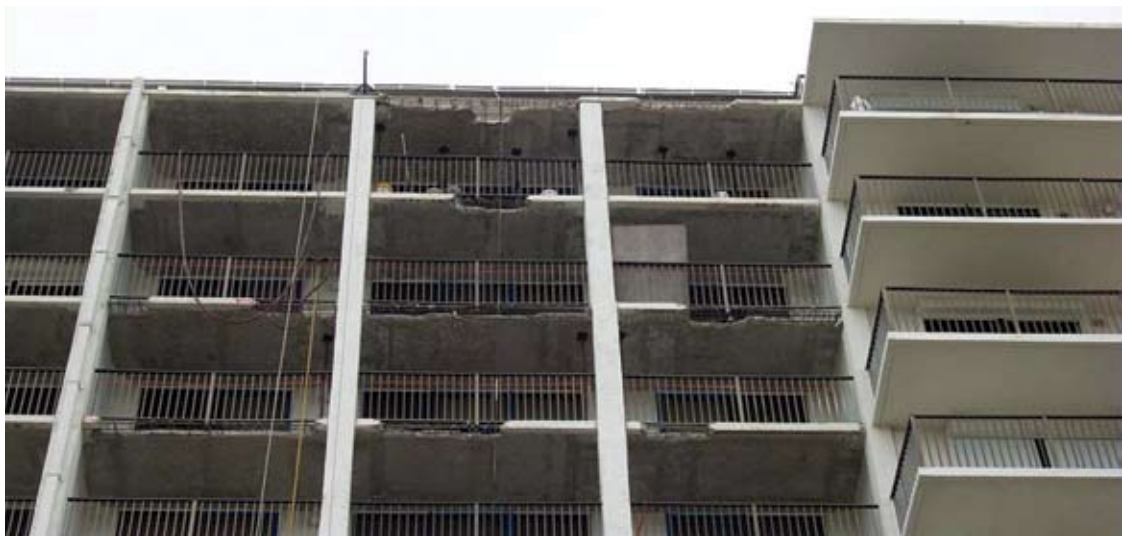
View of the stack and edge repair needed
