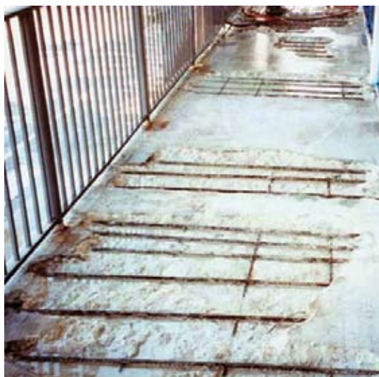
Typical balcony corrosion
