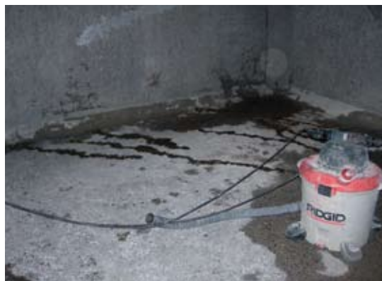
Front of tank showing major leaks
