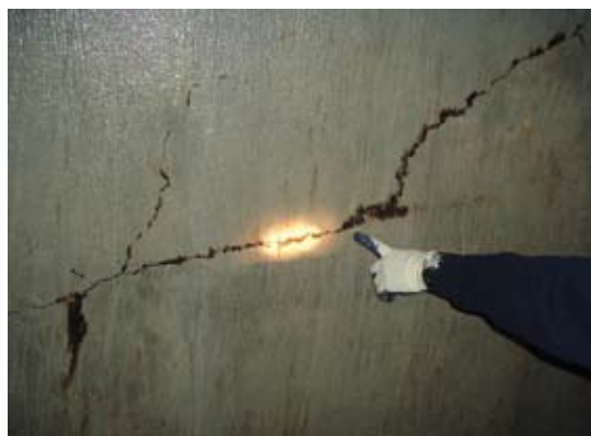
Leaking water tank
