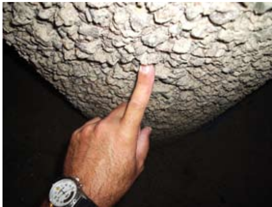
Close-up view of "soft" deteriorated concrete
