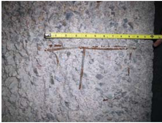
Corroded reinforcement showing through deteriorated concrete
