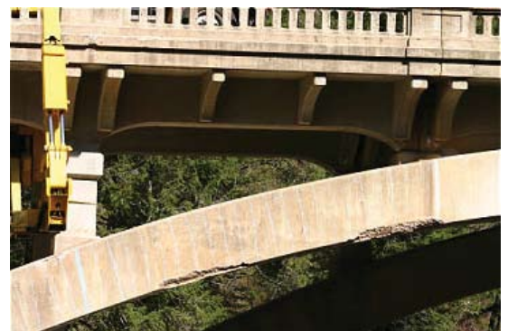
Fig. 2: Chloride-induced corrosion damage
