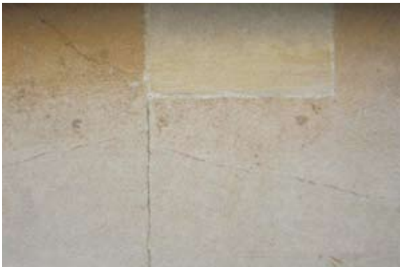
Aesthetic deterioration caused by the unsightliness of cracking of the stonework. Note the crack developing from a previous repair where the iron was not removed
