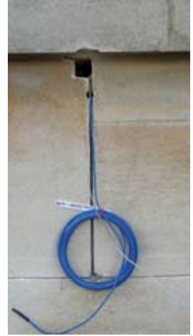
Position showing discrete breakout for drill and tap steel connections and reference electrode monitoring installation
