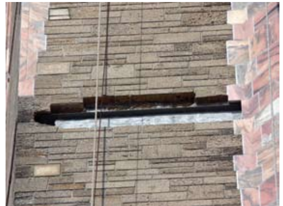
Coquina brick and underlying masonry had separated from tower
