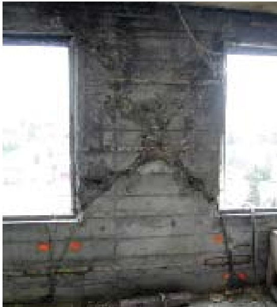
Fig. 1: Damage to walls caused by the earthquake
