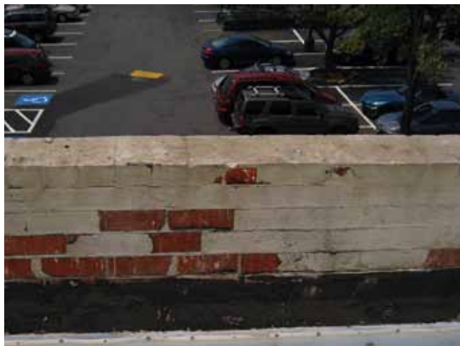
Brick faces are spalling off due to moisture infiltration and freezing-and-thawing damage
