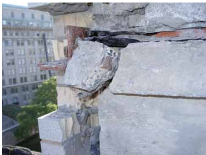
Expansion of brick façade and shrinkage of concrete frame has caused the concrete slab edge to shear off at a shelf angle embed
