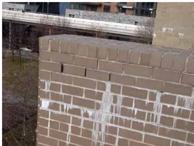
Efflorescence on face of masonry pier
