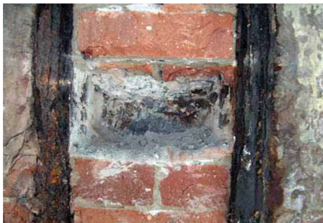
Structural steel column corrosion
