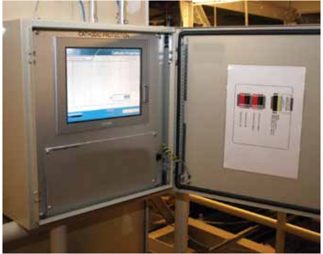
Monitoring equipment installed inside the building allows for remote monitoring and system adjustment
