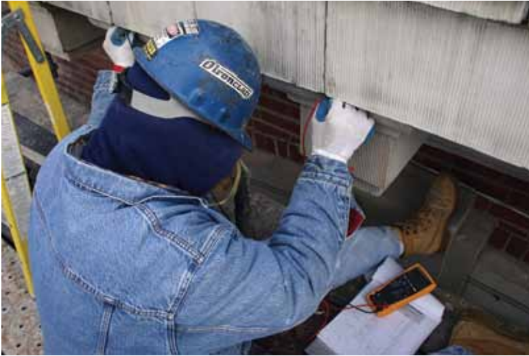
Continuity testing of impressed current cathodic protection system to be recorded on quality assurance tracking sheet in lower right of photo
