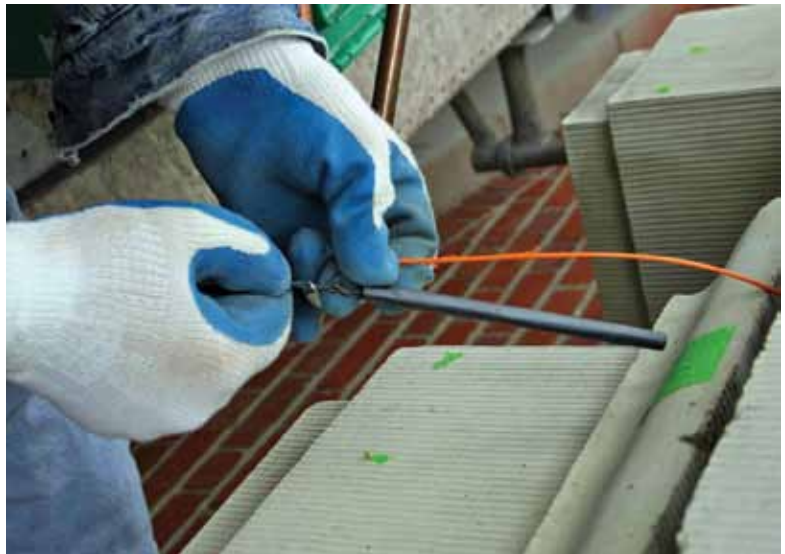
Discrete anode connected to power supply and ready for placement into mortar joint
