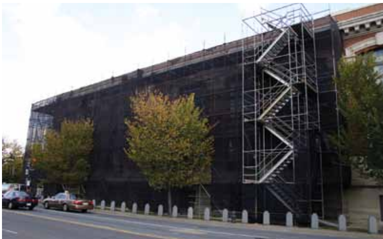
Access to top of building's cornice was provided by scaffolding for the overall façade restoration
