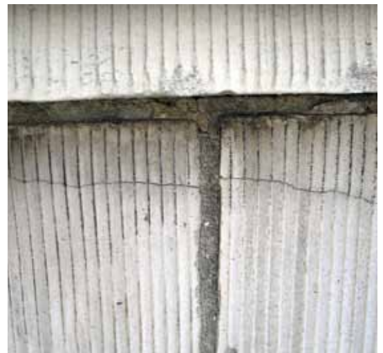
Damaged terra-cotta from corrosion of steel supports
