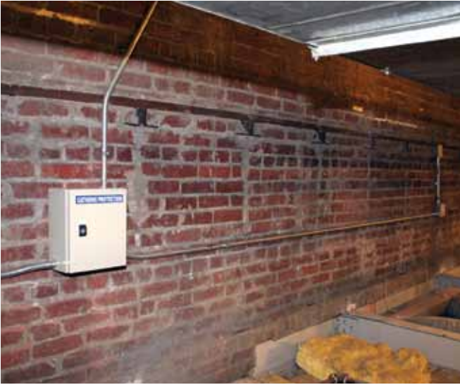
Power supply located in the interior of the building's attic space
