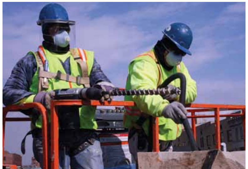
Anchorage holes were vacuumed after drilling to ensure they were clean so a proper bond could be formed with the anchor
