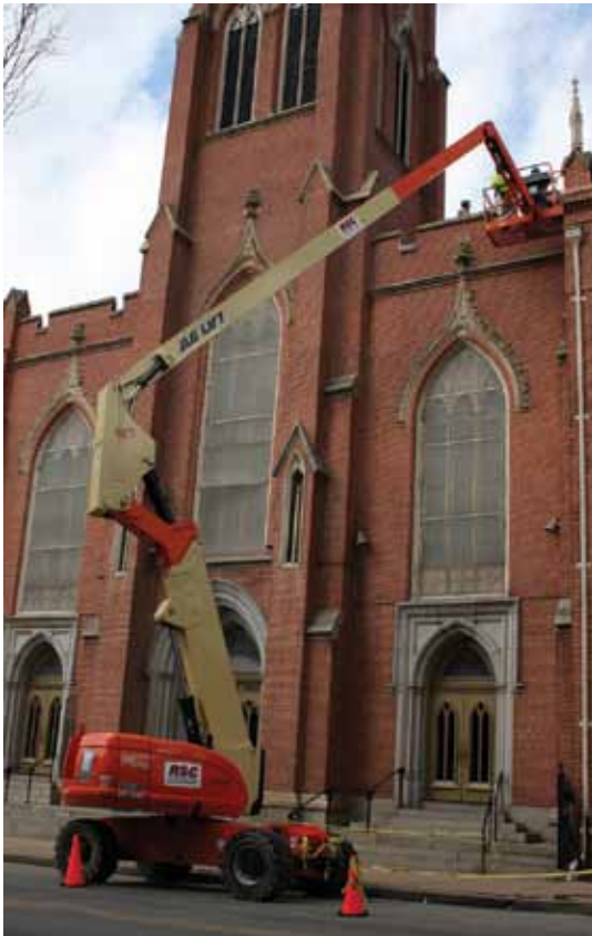
An 80 ft (24.4 m) boom lift was used for safe access to the work
