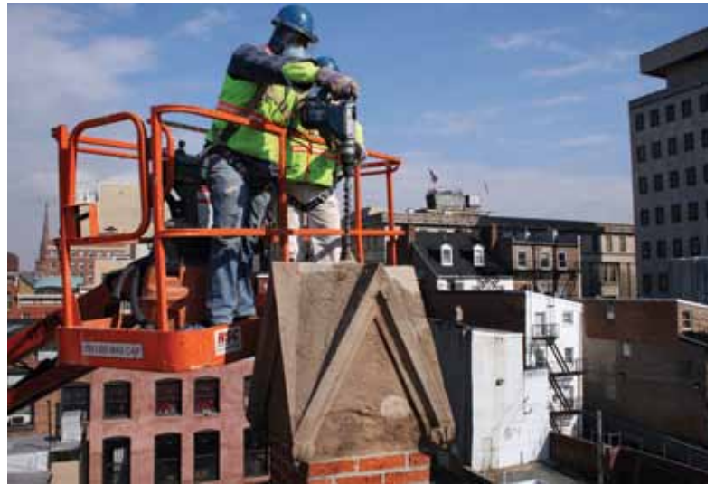
A cruciform bit was used to drill through limestone into masonry columns
