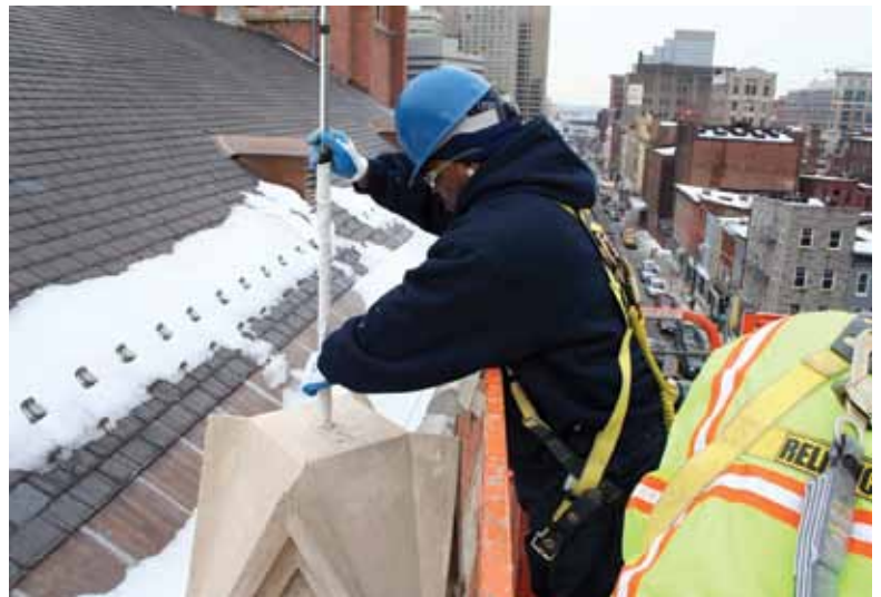
The 48 in. (1219 mm) long specialty anchor, covered in a long cotton sock to promote a good bond when the grout is pumped, is lowered into the anchor hole
