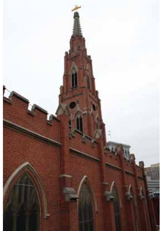
In the early 1900s, the church's signature spires were deteriorated to the point that they were a safety concern for pedestrians. They were removed, but never replaced
