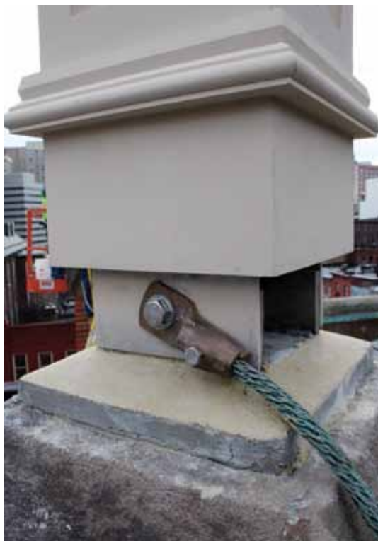
Lightning arrestor system attached to the stainless steel skeleton
