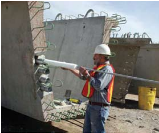
Fig. 2: U-shaped bridge girder (west end) and insertion of Styrofoam™ void prior to duct grouting
