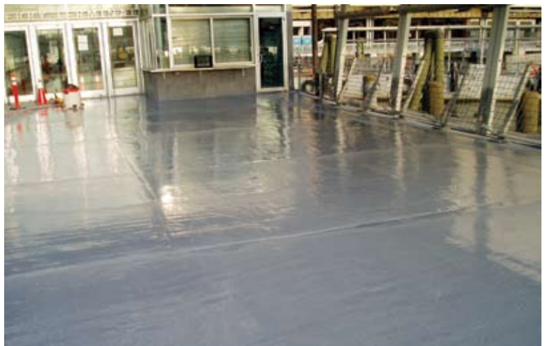
The completed area shines with the waterproof base coat, prior to the placement of the aggregate overlay lift
