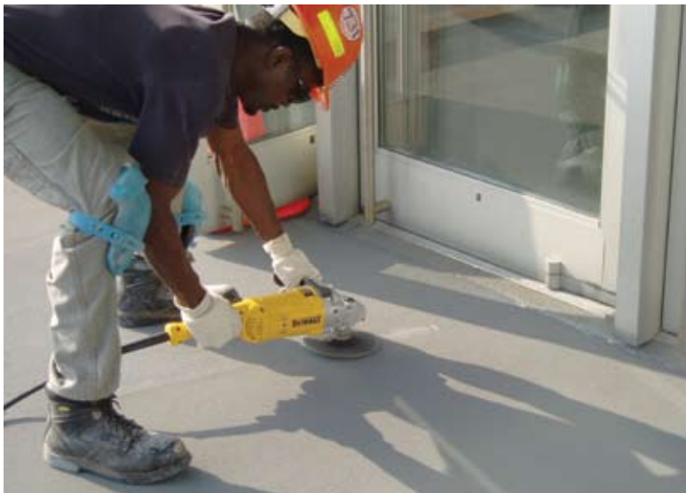
A crew member uses a grinder for minor surface detailing between overlay lifts
