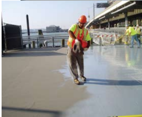
A pure polyurea-based aggregate reinforced broadcast overlay was placed over the entire surface in two lifts
