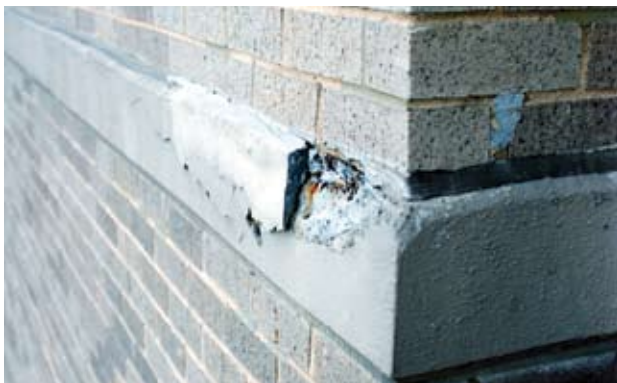
Failed concrete repair and failure in original adjacent concrete. Covered by warranty?
