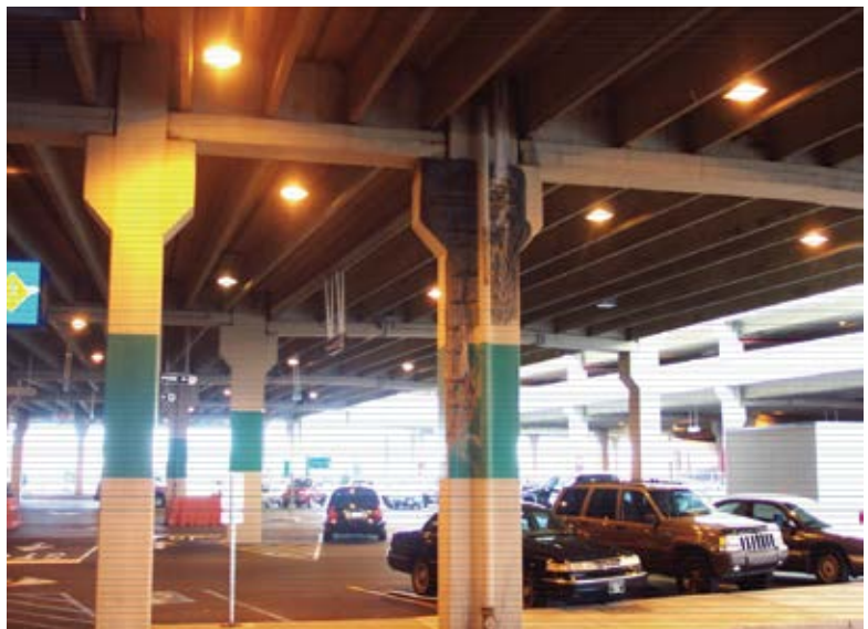
Fig. 4: Existing condition—vertical concrete column deterioration
