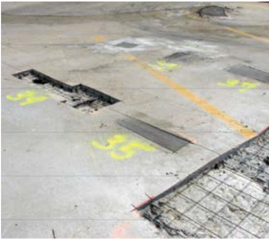
Fig. 7: Numbering of repair areas for documentation
