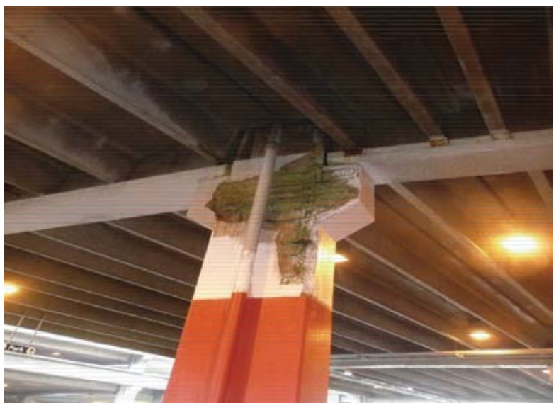
Fig. 5: Existing condition—vertical concrete column deterioration
