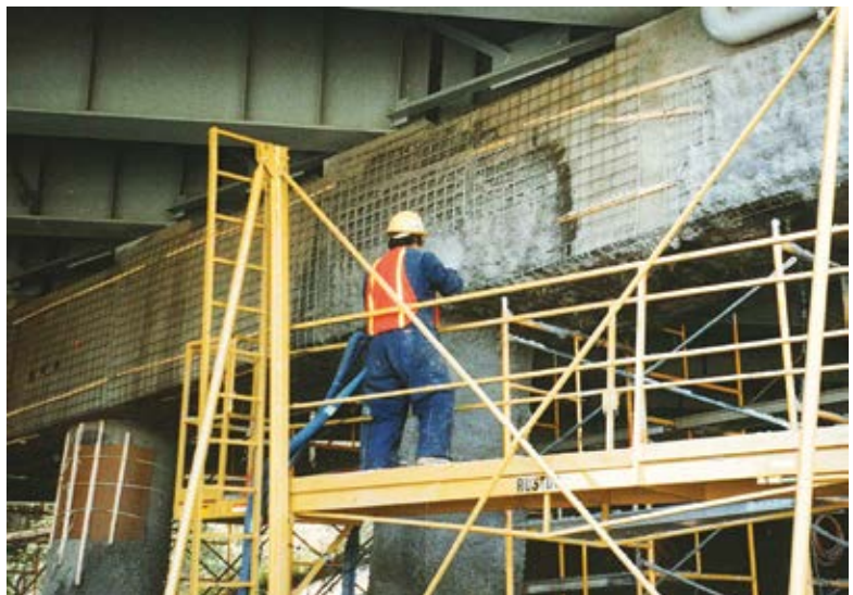
Fig. 4: Electrochemical chloride extraction
