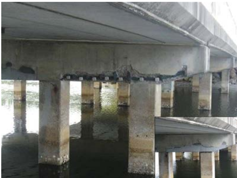
Fig. 4: Type 1A embedded galvanic anodes on bridge pier
