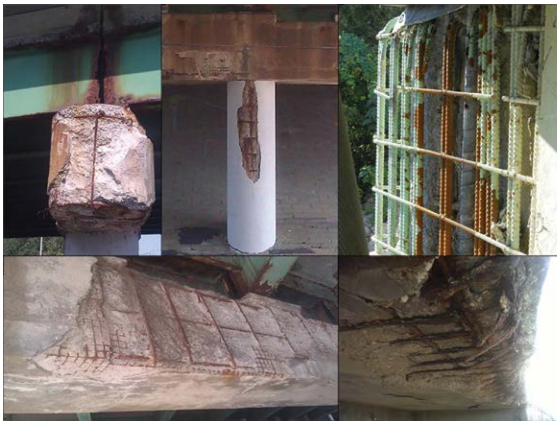
Fig. 1: Examples of steel corrosion on bridge structures
