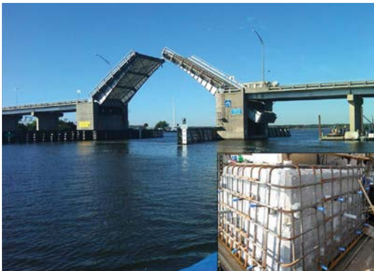
Fig. 3: ICCP system on bridge footing in marine environment
