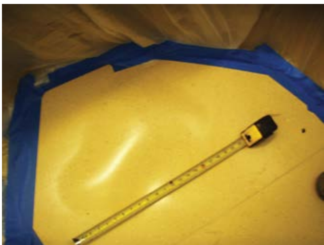
Fig. 4: Bubble in sheet vinyl flooring
