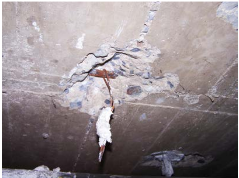
Fig. 3: Corroded tie connection to reinforcement
