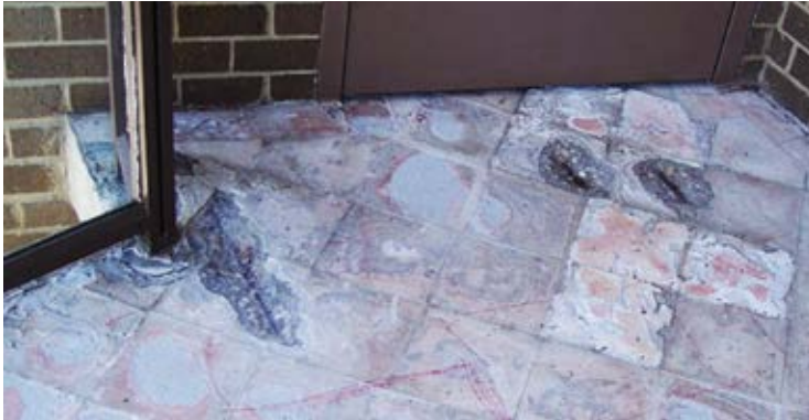
Fig. 1: Defects in existing concrete balcony
