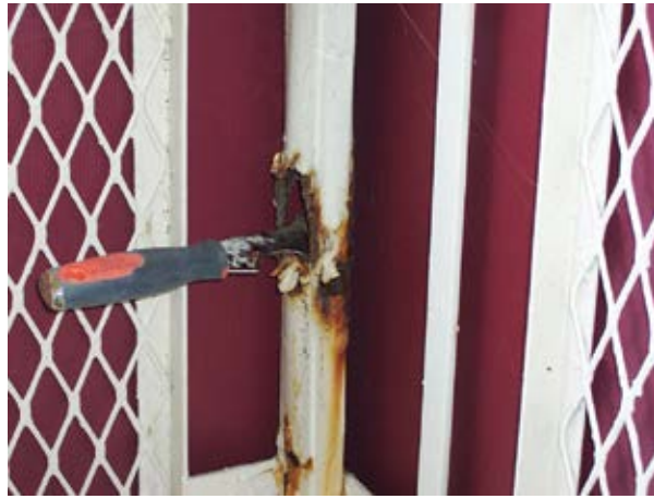
Fig. 11: Existing post with freeze damage
