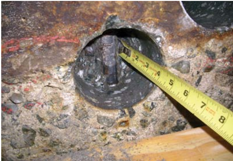
Fig. 6: Partial-depth core showing interior reinforcing steel with minimal corrosion stains
