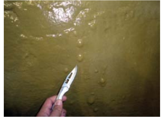
Fig. 12: Blisters in the protective coating
