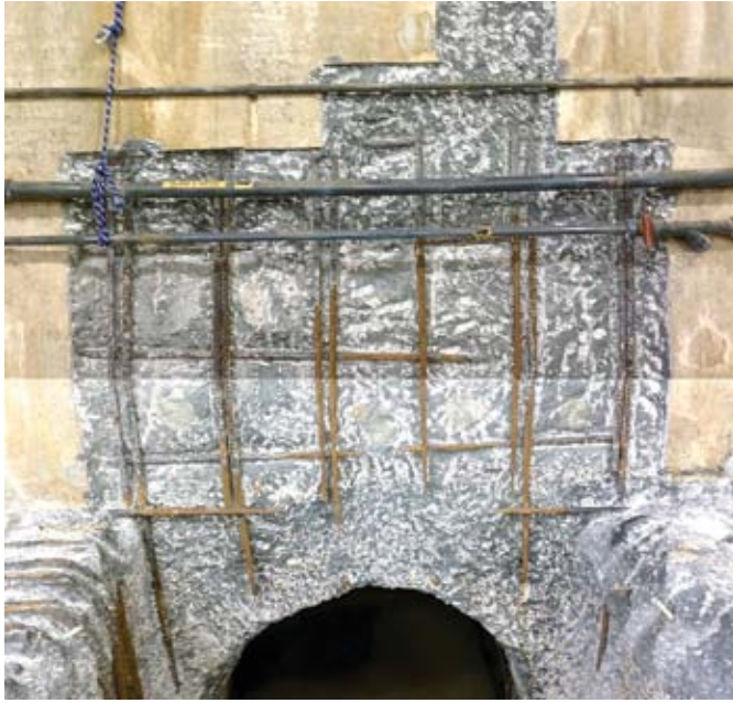
Fig. 10: Corroded reinforcing steel
