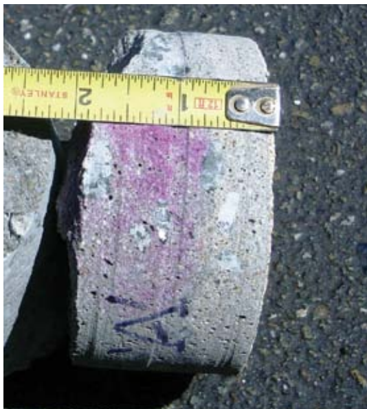
Fig. 7: Concrete carbonation depth of 0.75 in. (19 mm)
