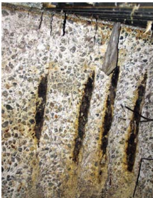
Fig. 5: Close-up view of concrete erosion and corroded reinforcing steel
