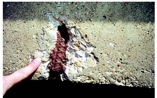
(Above and below) Corroded reinforcement of face of spandrel. Note the inadequate cover
