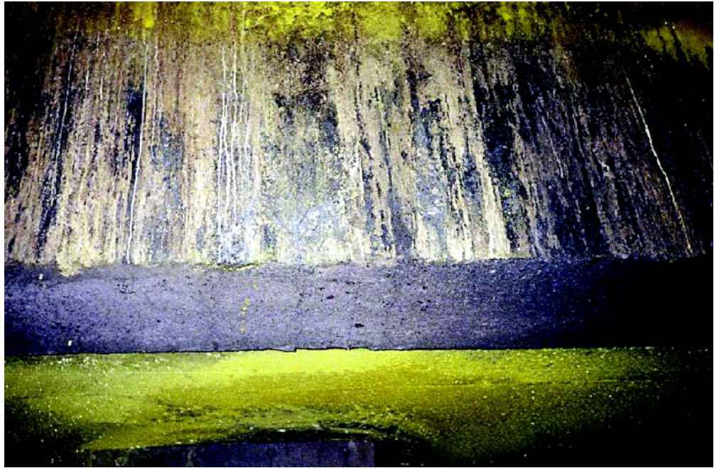
Figure 4: Area of repair in excellent condition after seven years of service
