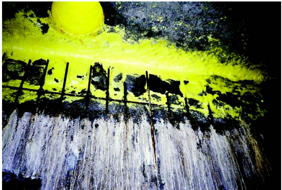
Figure 1: Exposed and corroded reinforcing steel in upper portion of wall
